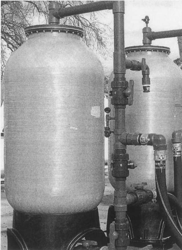
Figure 1. Perchlorate groundwater treatment system at Site-1 in California. Each resin canister was filled with \sim 120 gal of the bifunctional resin, Purolite A-530E, and typically ran at \sim 150 gpm.
