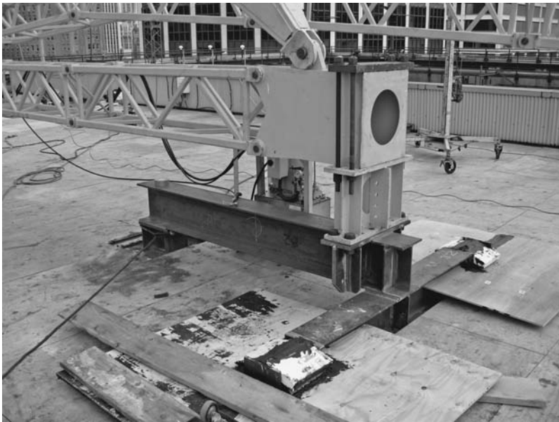
FIGURE 7.29 Sill end is connected to a relatively simple transfer that carries the load down to suitable building framing. ( Budco Rigging, Inc. )
