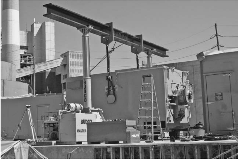
FIGURE 2.50 A simple telescopic gantry with two stocky lift cylinders, a header and a pair of lifting yokes, picking a piece of machinery by slinging around a pair of trunnions. ( Budco Rigging Co. )
