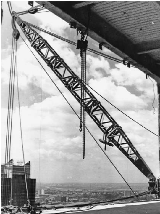
FIGURE 2.2 A 36-ft (11-m) Chicago boom installed at the McGraw-Hill Building in New York City during construction. The curved steel straps on the upper load block permit concentric mounting while allowing the derrick to boom in-to very small radii. The chain-fall in the foreground is for transferring loads from the derrick to the building floor. ( Lawrence K. Shapiro. )
