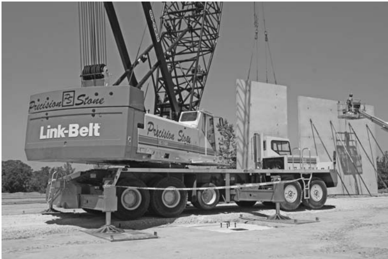
FIGURE 4.5 A truck crane with the cab overhanging the front outrigger. The crane may be restricted from lifting over the front quadrant unless the front outrigger is set in place, as in Figure 4.6. (Link Belt Construction Equipment Company.)
