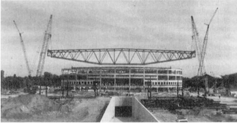
FIGURE 5.41 A double truss 290 ft (88 m) long and weighing 148 tons (134 t) being lifted by two crawler cranes with 160-ft (49-m) booms prior to traveling several hundred feet with the load. Including lifting attachments; each crane is carrying 84 tons (76 t), 88% of rated load, during this fully engineered and controlled lift. ( Douglas Steel Fabricating Corporation. )
