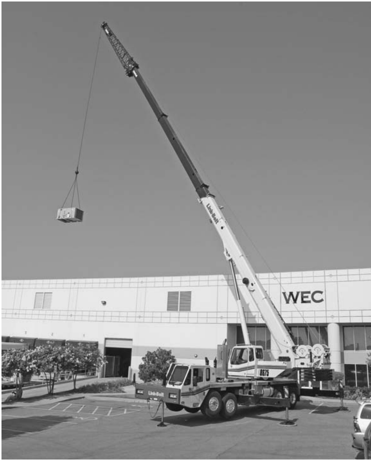
FIGURE 2.31 A 75-ton hydraulic truck crane lifting with a latticed extension lifting an air conditioning unit. ( Link Belt Construction Equipment Company .)
