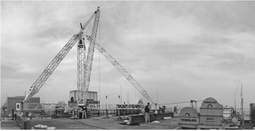
FIGURE 7.28 A rooftop stiffleg derrick. The mast is set directly above a column, but the two sills require large transfer beams. ( Budco Rigging Co. )
