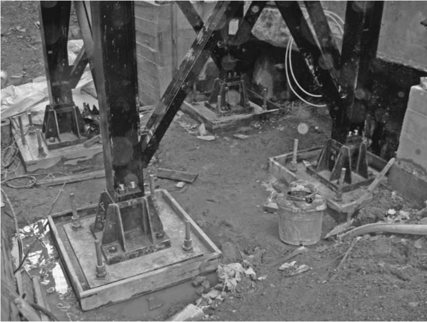
FIGURE 6.16 The foundation of this mast is comprised of an individual footing under each tower leg. The footings, in turn, are anchored to rock with the rock anchors tested and preloaded. Collectively the preload of the rock anchors must exceed the design uplift load of the respective leg. The bearing capacity of the underlying rock must be capable of supporting the combined preload and compression from the crane leg. ( Dominique Singh. )
