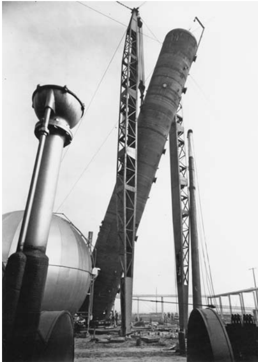
FIGURE 2.4 A pair of gin poles prepared for lifting a vessel. The tailing crane is not visible.
