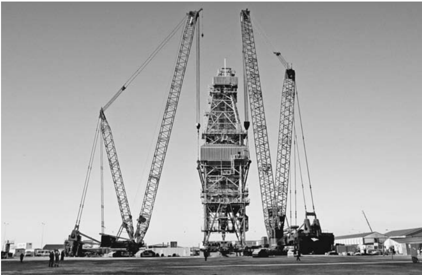
FIGURE 2.17 A two-crane lift with hammerhead-tipped booms. The hammerhead tips hold the load away from the boom by means of offset sheaves to permit the load to be raised clear of the booms. (Manitowoc Company, Inc.)
