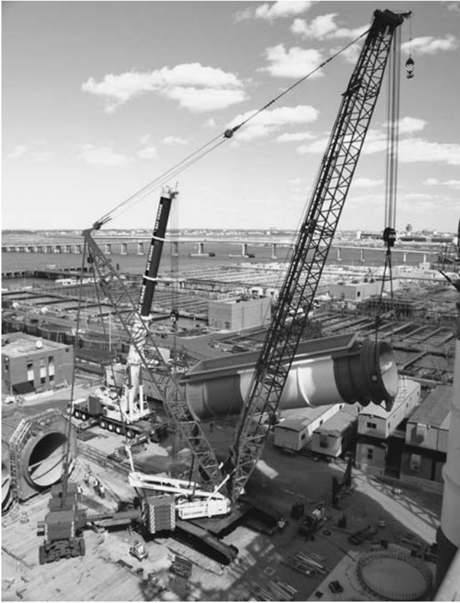
FIGURE 5.51 A two-crane lift of the configuration shown in Figure 5.46. The main crane, a Liebherr LR 1400 with a heavy lift attachment is attached to a trunnion. The tailing crane is a Liebherr LTM 1500. (Bay Crane.)
