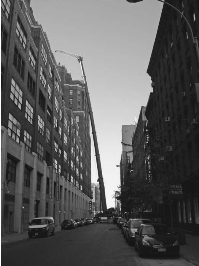
FIGURE 5.4 On a city street, a telescopic crane with an offset jib places mechanical equipment on the roof of a building. Clearance checking is needed if successful placement is not to be left to chance. ( Mathieu Chaudanson. )
