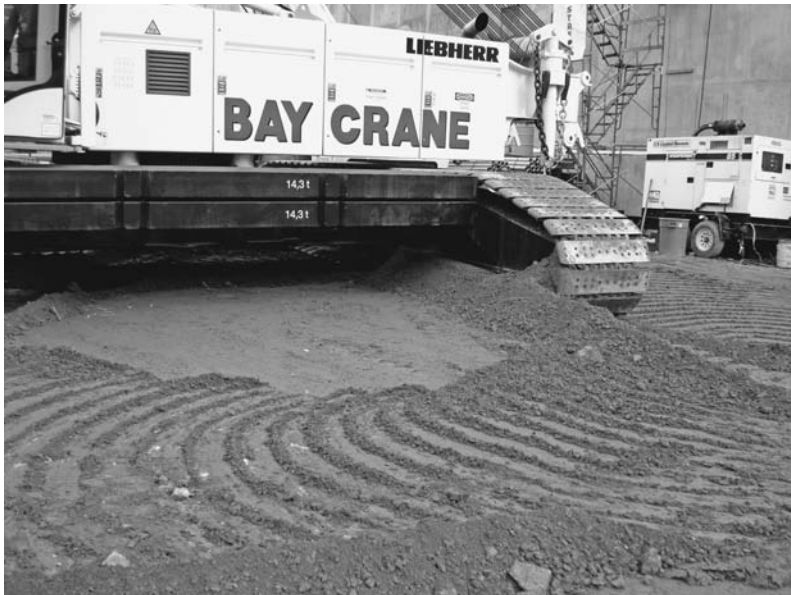
FIGURE 5.24 On firm level soil, a crawler crane can travel and sometimes operate without cribbing under the tracks. During a turning maneuver, the heavily loaded end of the track may gouge and push the soil. ( Mathieu Chaudanson. )
