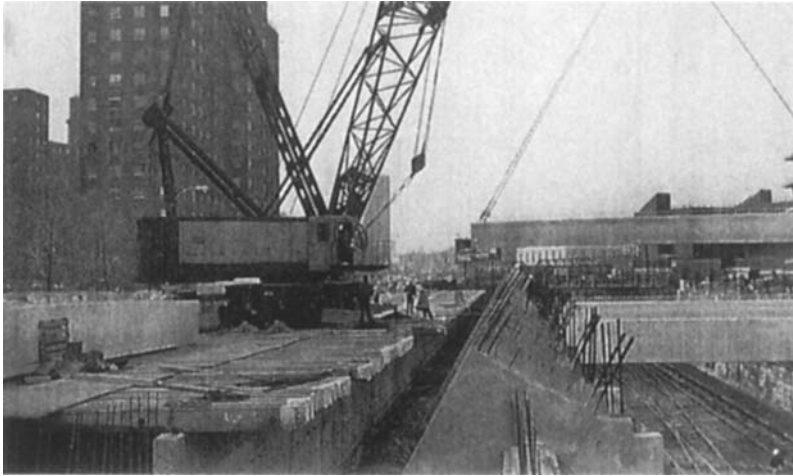
FIGURE 5.30 By using a heavy timber deck and placing the outriggers on the wall, it was possible to bring this 250-ton (227-t) truck crane close enough to place the precast girders shown. The line of steel plates was needed to spread wheel loads while moving the crane from one working position to the next at this project over the right-of-way of a commuter rail line.
