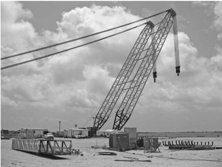
FIGURE 7.23 A mammoth-sized tandem gin pole for lifting vessels at a fabrication yard on the Gulf Coast. (Lawrence K. Shapiro.)
