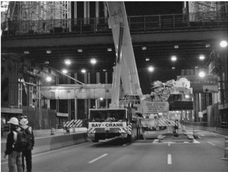
FIGURE 5.37 A 600-ton capacity telescopic crane set up for operation on the upper roadway of the George Washington Bridge. Special grillage frames were designed to carry the substantial outrigger loads to the main bridge girders below. Crane placements and outrigger reactions were carefully controlled to respect the structural limitations stipulated for the bridge. ( James Scheld. )
