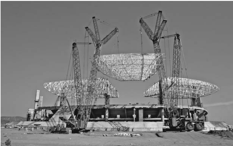
FIGURE 5.42 Pick of a space frame using a pair of Manitowoc 16000 crawler cranes equipped with the same front-end attachments but different heavy-lift counterweight arrangements. ( Manitowoc Corporation Inc. )
