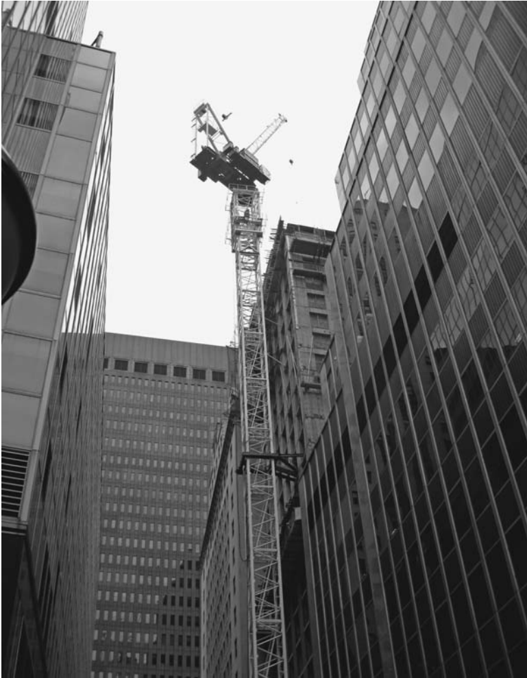
FIGURE 2.33 Pecco SN160 luffing boom tower crane at work as an external climber braced to the structure in an urban canyon of downtown Manhattan. The mast is braced to the building. Just below the crane superstructure is the climbing frame used to raise the crane for insertion of another tower section. (Lawrence K. Shapiro.)
