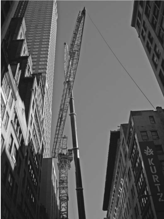
FIGURE 5.11 Tower-crane erection and dismantling are rigging projects where many of the most critical operations depend on maintaining clearance between the erection crane boom and the load. Placement of this hydraulic truck crane was controlled by adjacent buildings and by space needed on the street to assemble the tower-crane boom at a reach within the crane's capacity. (Paul Yuskevich.)
