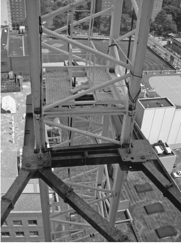
FIGURE 6.24 A collar and brace support an externally mounted tower crane. The collar, suspended from the mast with slings and turnbuckles, is very rigid to prevent the tower from distorting. ( Dominique Singh. )
