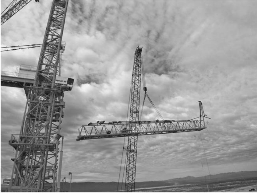
FIGURE 6.42 Erecting a tower-crane boom can entail tight clearances and drift even in open areas. ( Morrow Equipment Company. )
