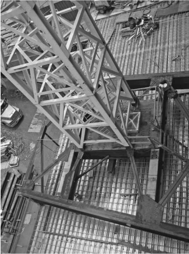
FIGURE 6.18 A steel base frame carrying the crane loads to building columns (not seen) and the foundation wall. The base frame has plan braces to resist slew torsion and lateral loads. ( Dominique Singh. )
