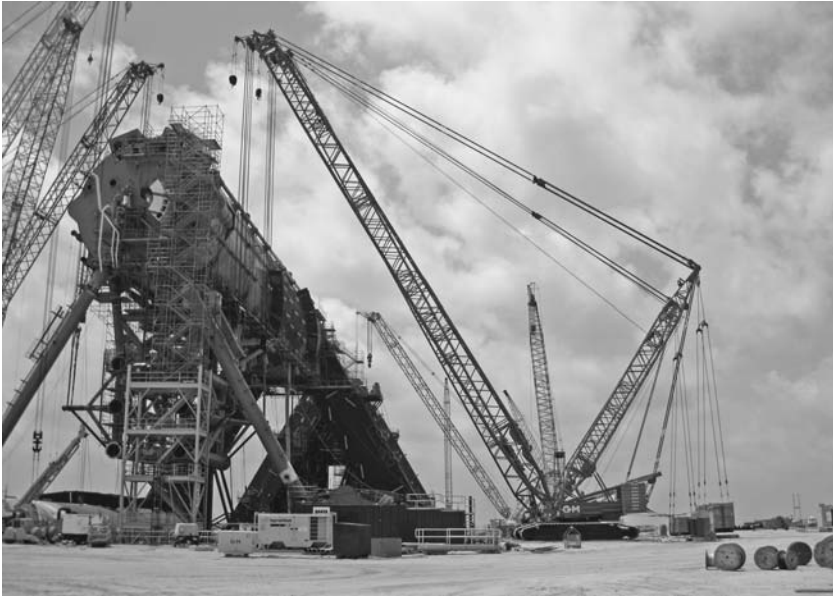
FIGURE 2.27 A Demag CC2800 crawler crane with live mast and a tray of auxiliary counterweights suspended from it. The enhanced capacity of the arrangement is needed for heavy lifting assembling this offshore oil platform. (Lawrence K. Shapiro.)
