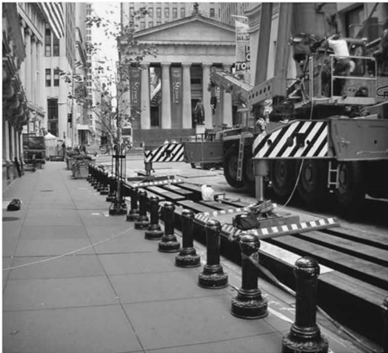
FIGURE 5.23 Two-tiered cribbing of plates and beams required to spread the outrigger loads over a wide area due to the presence of a subway line under the sidewalk and vaults under the sidewalk in front of the New York Stock Exchange. ( Mathieu Chaudanson. )
