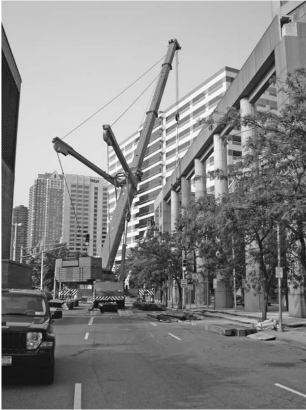
FIGURE 2.25 Liebherr LTM 1500 telescopic truck crane with a guy attachment dismantling a heavy structure. The guy attachment stiffens the boom, increasing its structural limitations. ( Mathieu Chaudanson. )
