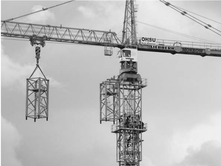
FIGURE 2.41 A hammerhead tower crane using a suspended tower section as a balancing weight for climbing. There is another tower section hung from the climbing trolley, poised for insertion below the superstructure. ( Morrow Equipment Company. )
