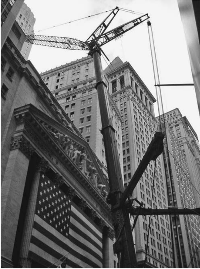
FIGURE 2.22 Liebherr LTM 1500 telescopic truck crane at the New York Stock Exchange lifting mechanical equipment on the roof with the luffing jib. With the help of the guy attachment, visible on the back of the boom, this configuration offers high lifting capacity reaching far over the front façade. ( Jay P. Shapiro. )
