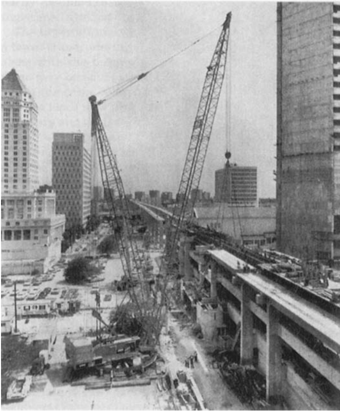
FIGURE 2.26 A Manitowoc 4100 W crawler crane, fitted with a Ringer attachment, at work on Metrorail in Dade County, Florida. Note that the boom and live mast are stepped onto a carrier riding on the large-diameter ring that constitutes the machine's tipping fulcrum. The added concrete counterweight blocks also ride on the ring. The mast gives the boom added structural capacity, while the additional counterweight and the placement of the tipping line well in front of the machine increase its stability. (Manitowoc Company, Inc.)
