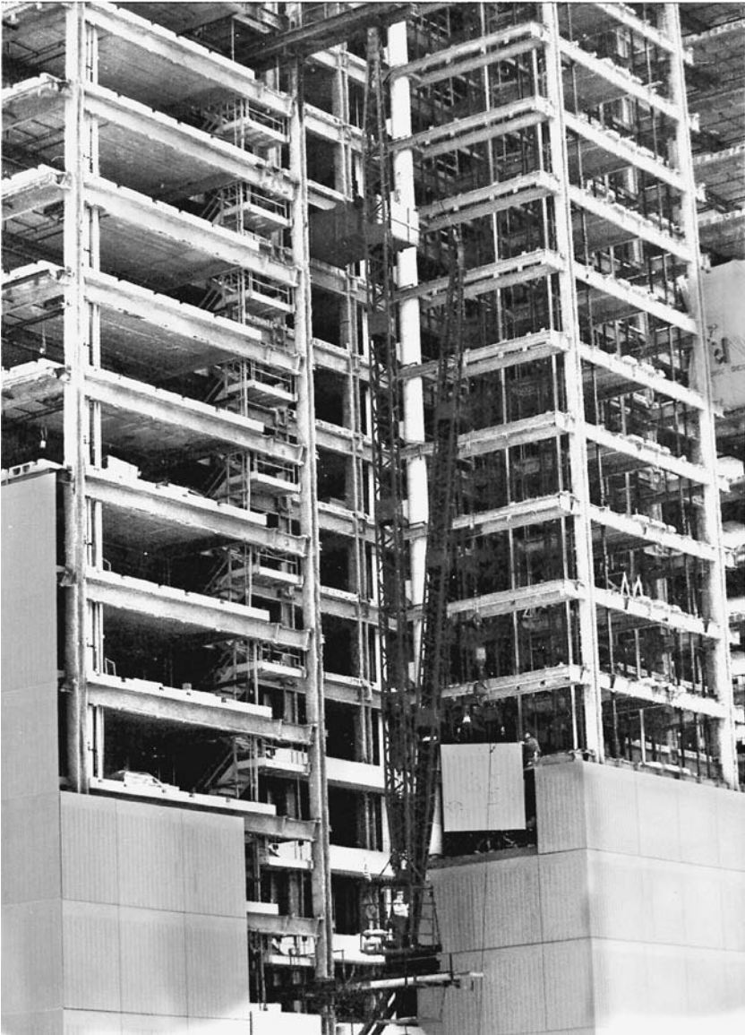
FIGURE 2.7 A column derrick used to place heavy precast facing panels on a high-rise hotel under construction. This is a guy derrick without guys, a concept of A. J. McNulty & Co., Inc., designed by the authors' firm. The upper support (which replaces the guys) and the base support are cantilevered from the building frame. (A. J. McNulty & Co., Inc.; photo by Robert Weiss.)
