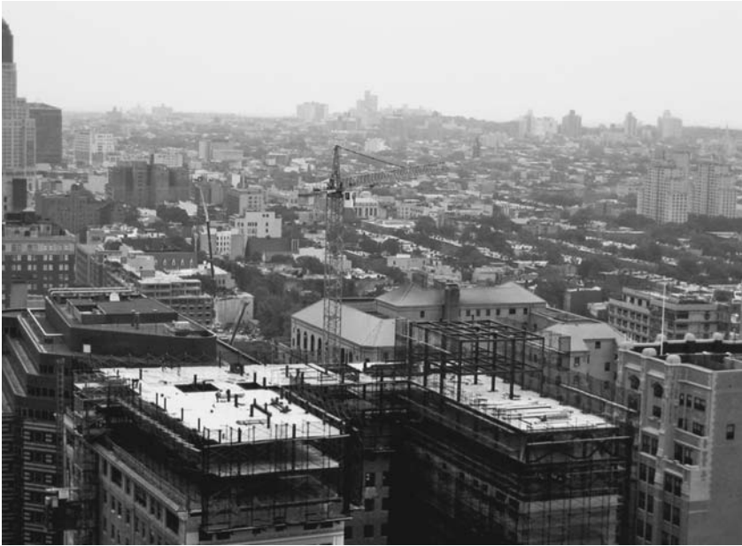
FIGURE 6.17 This crane is supported on a steel base built into existing roof framing. The crane is erecting new steel to add floors. The building requires shoring and reinforcement to carry the crane loads. ( Lawrence K. Shapiro. )
