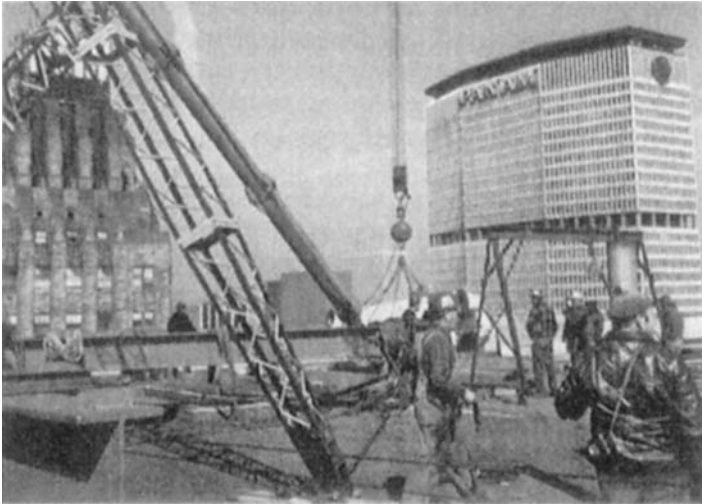
FIGURE 7.24 The very light duty gin pole in the foreground is used to erect and dismantle the stiffleg derrick seen in part. For the small loads involved, the pole is seated on a piece of planking located above a roof beam, and wire-rope ties are used to stabilize the pole foot. (Lawrence K. Shapiro.)
