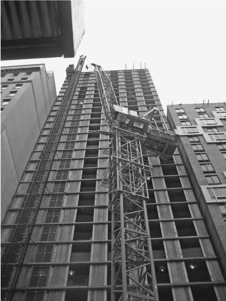
FIGURE 6.3 A top-climbing tower crane partly jacked down after completion of its work. It cannot swing around, but is able to swing enough for the boom to clear the hoist mast to the left. ( Lawrence K. Shapiro. )
