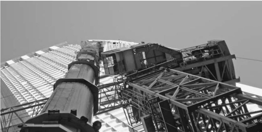
FIGURE 8.2 Telescopic mobile crane dismantles a luffing jib tower crane in an urban setting. The tower crane has a limited ability to swing because the newly erected building is in the way, and the position of the mobile crane is constrained by the limited space of the narrow city street. As can be seen, the operation must be carefully planned and communicated to the field crew. ( Mathieu Chaudanson. )
