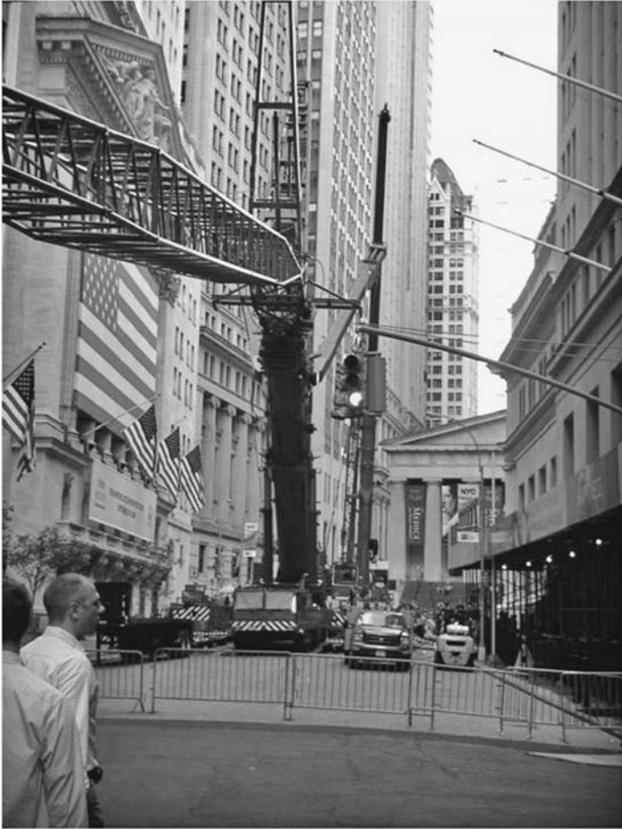
FIGURE 2.23 Liebherr LTM 1500 telescopic truck crane with the luffing jib being raised up after assembly on a city street. The luffing jib is out in front of the retracted boom; its tip has a wheel that allows it to be rolled on the ground as the boom is raised. When the angle between the boom and jib is 90^\circ , the jib tip is lifted off the street. After the jib is fully aloft, the boom is telescoped as needed. (Jay P. Shapiro.)
