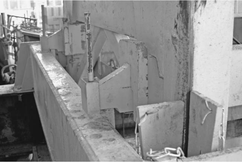
FIGURE 6.32 Working dog on a Potain internal-climbing tower crane, resting on the beams of the climbing base. The dogs retract when the crane is jacked up. Wedges for lateral support are visible in the near corner. ( Manitowoc Corporation Inc. )
