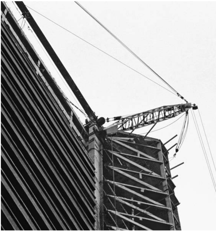
FIGURE 7.4 Chicago boom clamped to the weak axis of a column and arranged for landing loads to the left. Several parts of line are used in the right swing line to develop enough force to pull the boom away after unloading. ( Gendelman Rigging and Trucking, Inc. )
