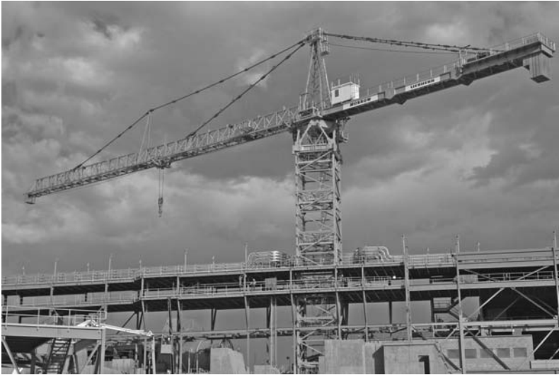
FIGURE 2.40 A 2000-tonne-meter tower crane freestanding on an industrial site in Mexico. The tower sections, too large for conventional trucking, are designed to be broken down into small pieces. ( Morrow Equipment Company. )
