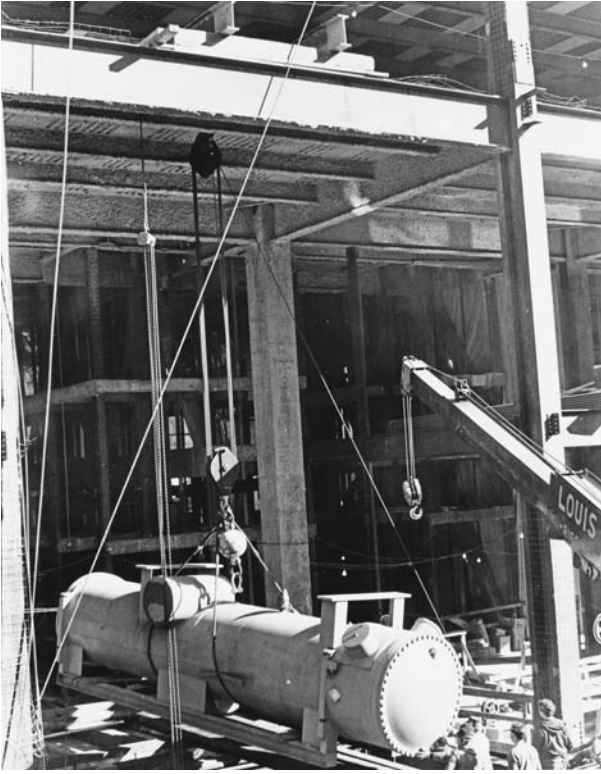
FIGURE 2.8 The bottom element of a large air-conditioning chiller ready to be lowered into a subcellar by a shaft hoist. The unit was rigged over the opening on steel beams, which will be removed by the small telescopic crane. The 30-ton (27-t) machine was one of several installed at the McGraw-Hill Building. (Lawrence K. Shapiro.)
