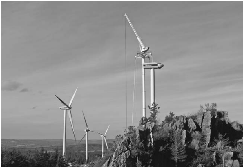
FIGURE 8.3 A wind turbine being erected in Spain by a unique self-erecting tower crane designed for this purpose. Planning and coordination must be extensive to set up such a massive crane in a remote mountainous site. By nature, this is a major lifting operation. ( Manitowoc Corporation Inc. )
