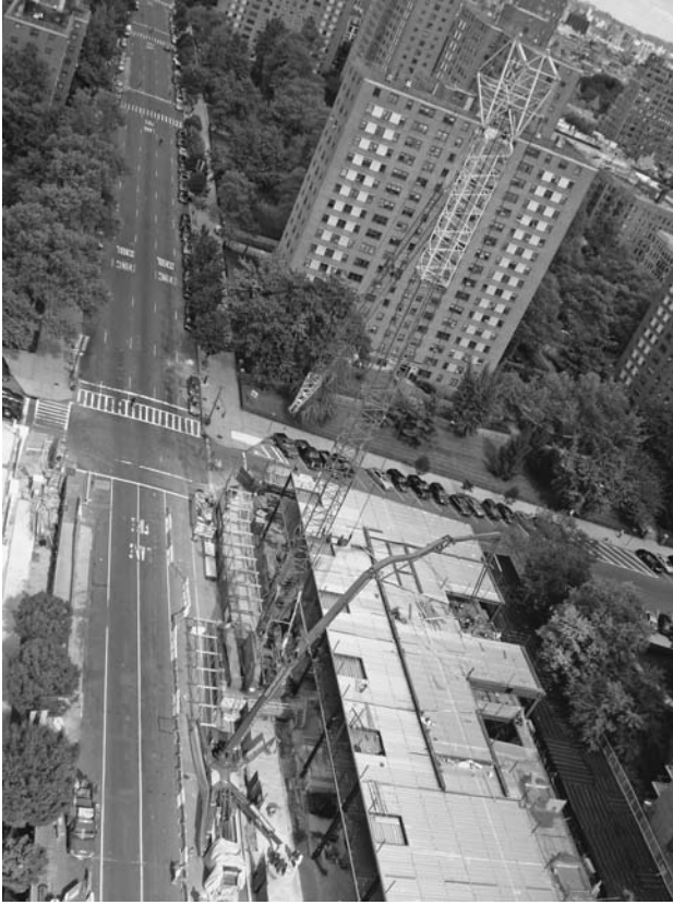
FIGURE 2.24 A crawler crane with a tower attachment. The boom is folded down in an out-of-service position. The boom is not working because the concrete placing boom in the foreground is in operation. ( Mathieu Chaudanson. )
