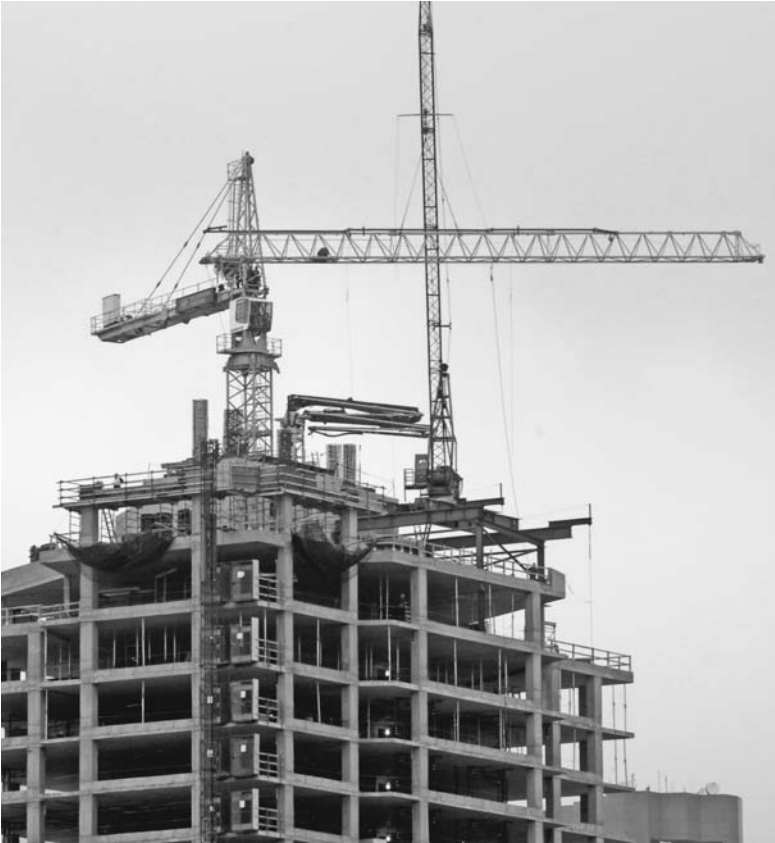
FIGURE 6.29 This internal-climbing crane is supported in the building. It must now be disassembled and lowered to the ground by the other roof-mounted crane. (Morrow Equipment Company.)
