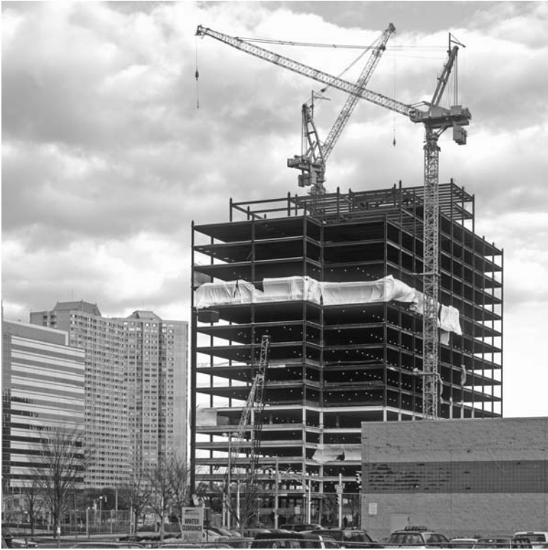
FIGURE 6.2 Luffing boom tower cranes erecting a steel-framed building. The luffing motion helps avoid boom and hook interferences. Coordination is much easier than in Figure 6.1, but communication among operators is still important. ( Morrow Equipment Company. )
