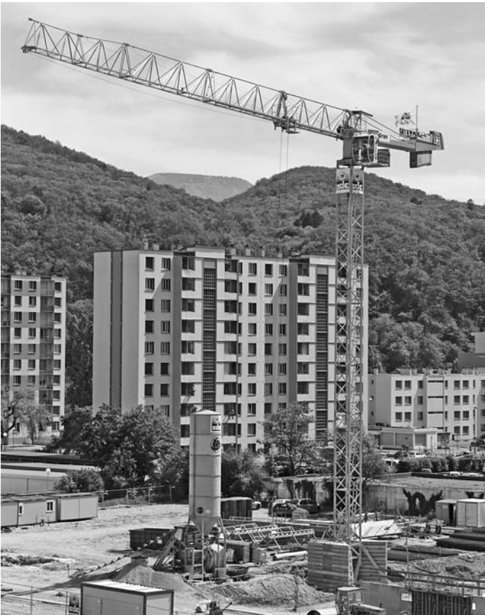
FIGURE 2.39 A hammerhead tower crane of the flattop style, freestanding on a chassis base stabilized with ballast. ( Manitowoc Company, Inc. )
