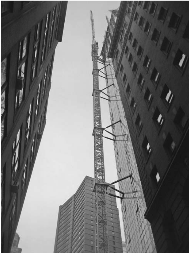
FIGURE 6.22 A crane braced to the outside of a high-rise reinforced-concrete building. Curtain wall is erected around the tie struts. During the jacking-down operation, the struts must be removed without causing damage to the delicate wall system. (Dominique Singh.)
