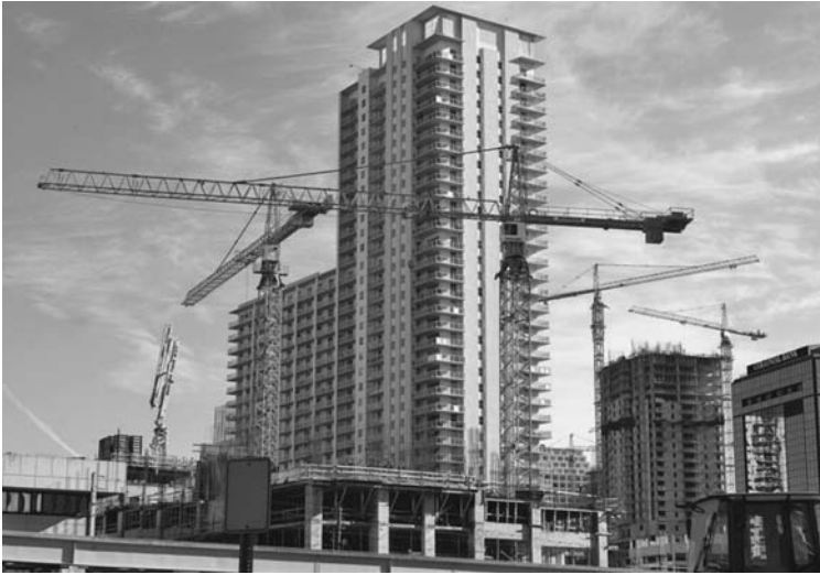
FIGURE 6.1 Tower cranes with overlapping operating areas require careful planning, field coordination, and operator attention. The site in the foreground has a concrete placing boom that must not be allowed to interfere with the two nearby tower cranes. ( Morrow Equipment Company .)
