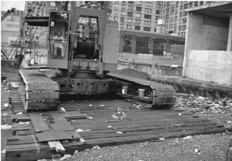
FIGURE 5.26 Timber mats were used here to level out the crane working area while also spreading track loads over a wider bearing area and permitting some travel. Plywood is placed over the timber mats for leveling. (Lawrence K. Shapiro.)
