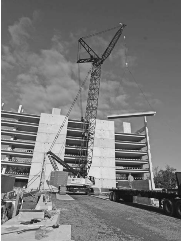
FIGURE 5.6 A 300-ton Link Belt 348 HYLAB 5 with a luffing jib erecting a precast concrete parking garage. The boom tip is higher than the building, so the entire range of motion for the jib is in the clear. ( Link Belt Construction Equipment Company. )
