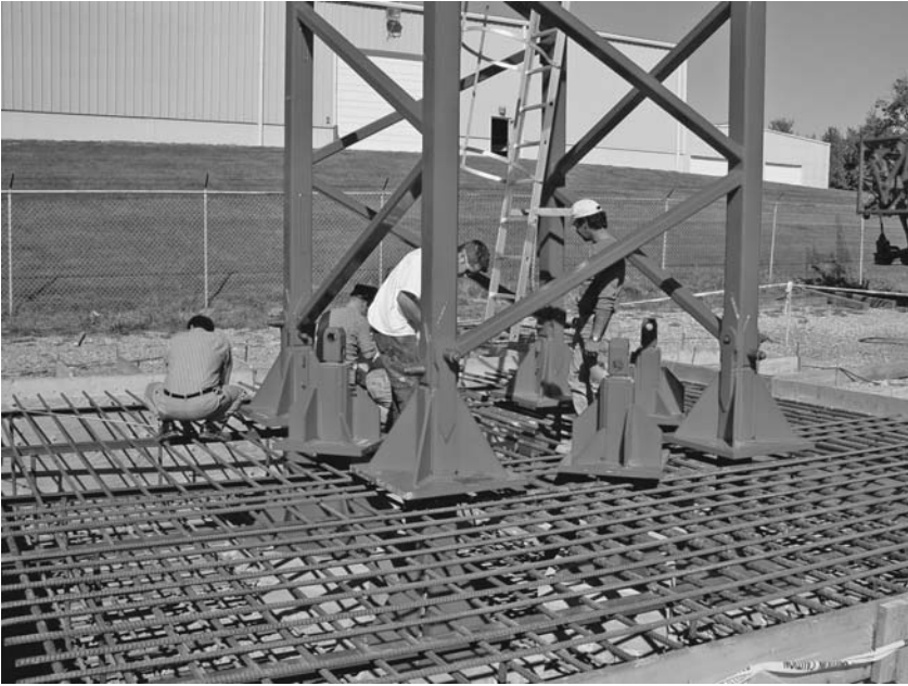
FIGURE 6.5 Tower-crane spread footing under construction with expendable legs visible under the tower section and rebar mat. The tower section is used as a template to assure proper alignment of the expendable legs and to allow the mast to be plumbed before the footing is poured. The footing mass provides ballast for resisting overturning moment. (Manitowoc Corporation Inc.)
