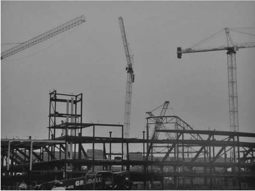
FIGURE 3.1 Havoc wreaked on tower cranes by a squall known as a bow echo front. The cranes were at work when the storm struck without warning. (Lawrence K. Shapiro.)
