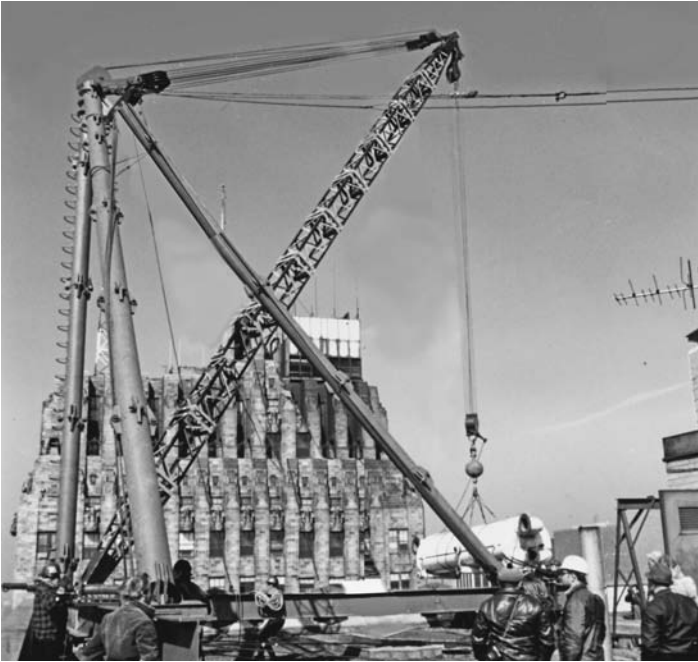
FIGURE 2.5 Stiffer derrick with a 62-ft (19-m) boom lowering part of an air-conditioning chiller. This derrick of 35-tons (32-t) capacity is made up of short-pinned components so that it can fit into elevators or jobsite material hoists. Both derrick and installation were designed by the authors' firm. (Lawrence K. Shapiro.)
