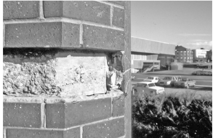
Figure 29 Brick slips failed at face of concrete floor
