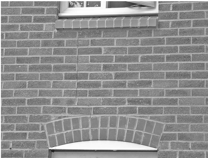
Figure 21 Structural cracking of concrete brick masonry resulting from the lack of design detail (expansion joint) in a long 'run' of brickwork. Cement-based masonry products typically shrink during the first few months of use, and the design of masonry structures needs to take this into account
