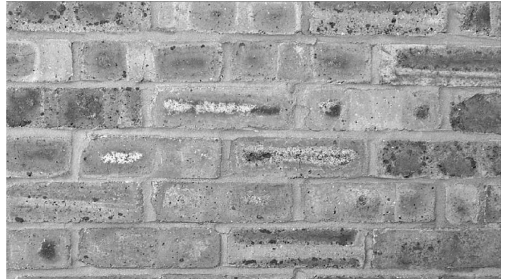
Figure 12 Efflorescence resulting from the formation of black cores and surface reduction markings (black areas) on 60-year-old Staffordshire Coal Measure Shale common bricks
