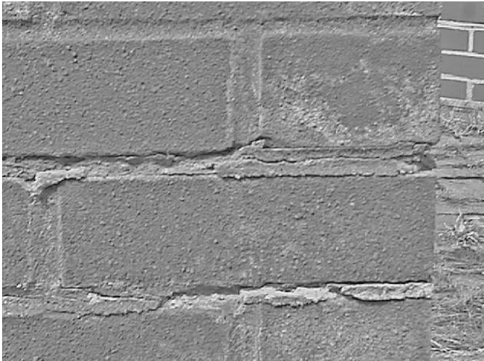
Figure 22 The effects of sulfate attack on cement-based mortar. The 'tooled' joint is often cracked along the centreline and behind the mortar is very soft and 'mushy'. Expansion of the mortar commonly results in the deformation of the masonry structure and, when seen in chimneys and boundary walls, often results in the need to rebuild the structure
