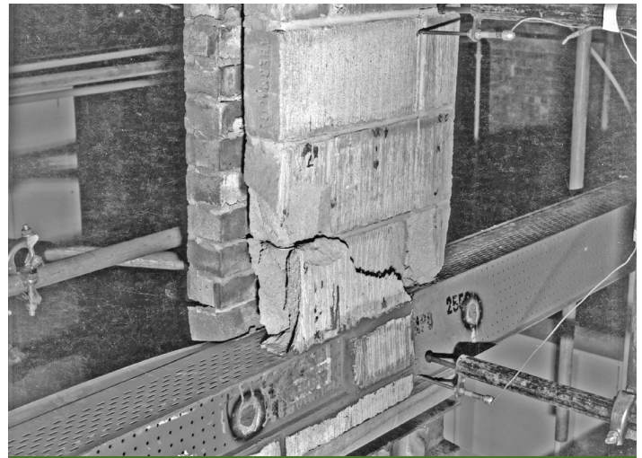
Figure 25 Local failure of a lintel bearing
