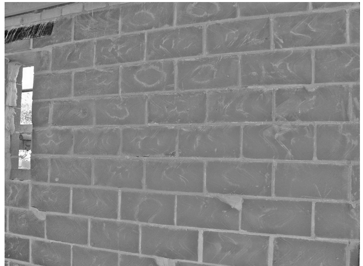
Figure 13 An example of internal insulation blockwork showing the deposition of water-soluble salts during the construction phase
