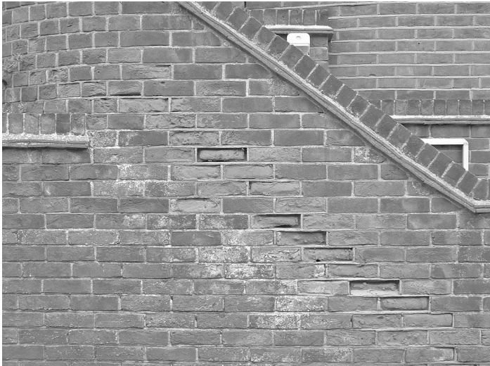
Figure 6 Frost damage due to the localised conditions of use. The damaged bricks here follow the position of the flight of steps on the other side of the wall. The bricks are therefore exposed to a higher level of saturation than the rest of the wall
