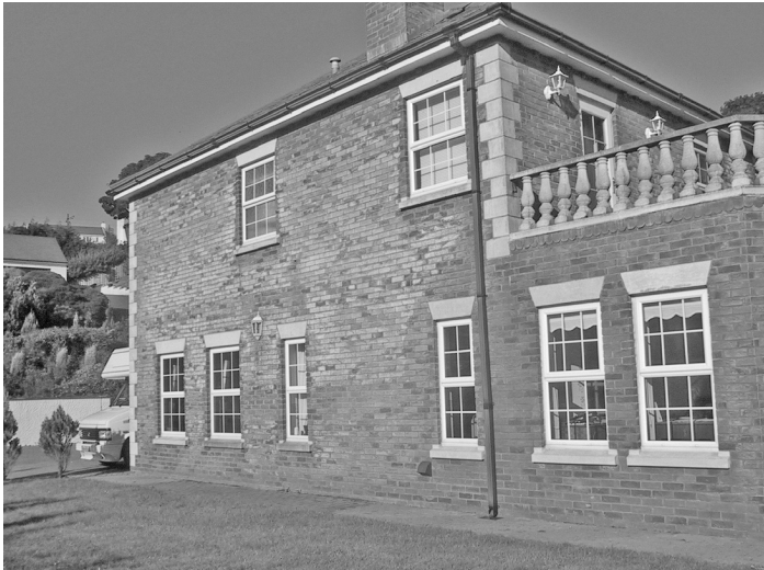
Figure 11 Efflorescence, commonly associated with the movement to the surface of the brickwork of water-soluble sulfate salts, in this case potassium sulfate
