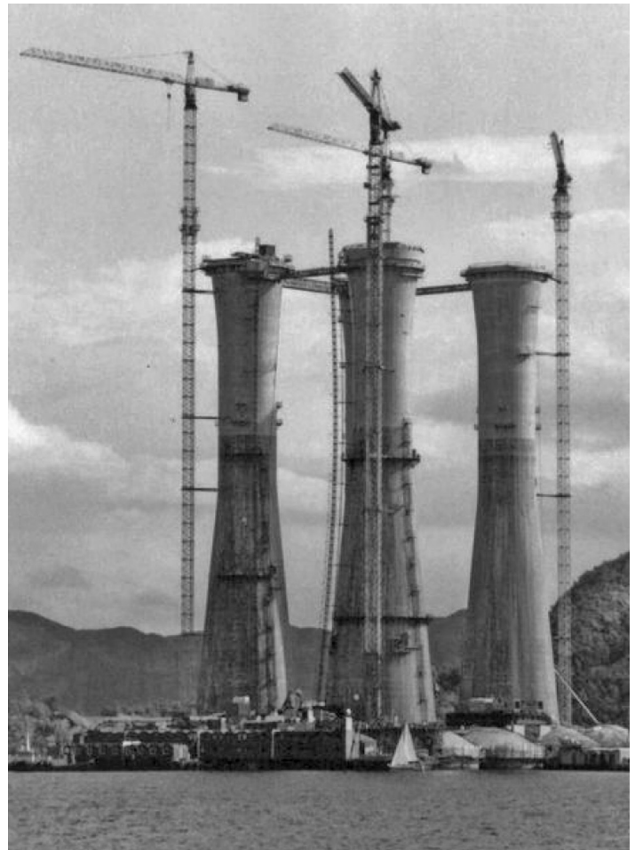
Figure 2 The Troll A platform was built over a period of 4 years, using a workforce of 2000. With a total height of 472 m, Troll A was the largest structure ever to be built and moved. The total weight when launching was 1.2 million tons. A total of 245 000 m 3 of concrete and 100 000 tons of steel for reinforcement were used. The amount of steel corresponds to 15 Eiffel towers. The platform was placed at a depth of 300 m. For stability, it is dug 35 m into the sea floor
