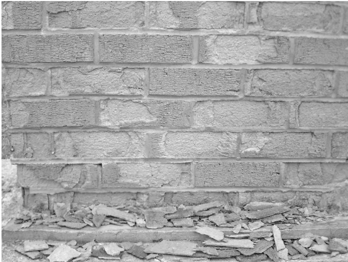
Figure 4 An example of the 'classic' delamination failure due to cyclical frost action on a free-standing wall. In extreme cases the face of the brick comes off as a single 'brick slip'
