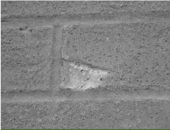
Figure 16 Spalling/chipping as a result of the action of water ingress into a hairline crack and subsequent frost action propagating the crack to the point of the total loss of bond. The original hairline crack was more than likely a result of mechanical impact
