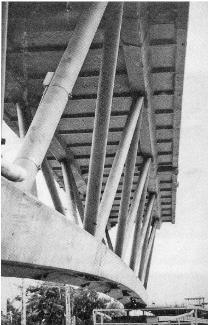
Figure 6 The Sherbrooke Footbridge in Sherbrooke, Quebec, spans 60 m across the Magog River with a precast truss made of reactive low quality powder concrete. The deck slab is 30 mm thick and 3.3 m wide. There are stiffening ribs, 100 mm wide by 70 mm deep, on the two edges of the beam and transverse ones every 1.25 m. These stiffening ribs had internal prestressing for purposes other than load capacity
