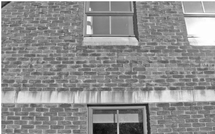
Figure 8 Bricks from mainland Europe which have a similar firing characteristic as the Weald bricks in the UK. In this case the iron and manganese compounds have become mobile and have been deposited on the face of the bricks, mortar and stone string course
