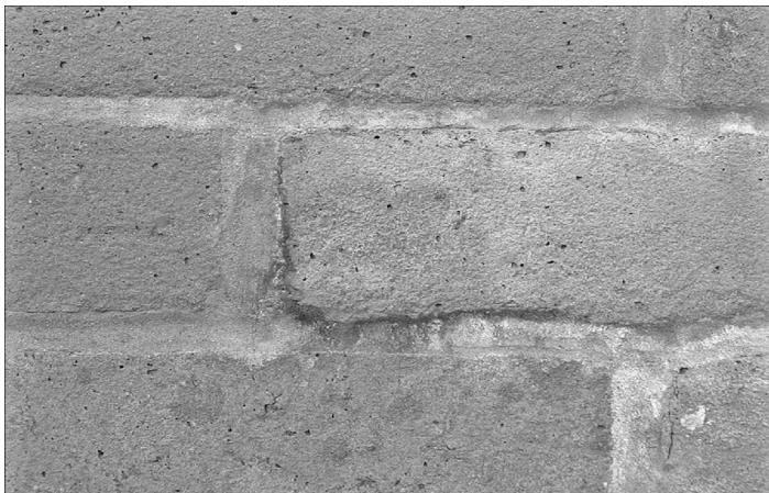
Figure 9 Deposition of iron staining on mortar joints as a result of a pH change in the transportation solution
