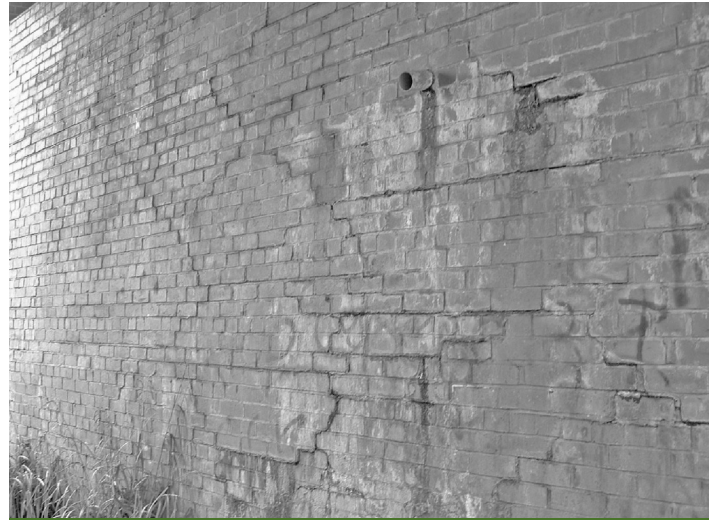
Figure 23 Railway bridge masonry faced abutment with major structural cracking resulting from the formation of sulfate attack and formation of thaumasite. The source of the sulfate, in this case, is almost certainly from the use of 'cinders' and furnace bottom ash/clinker
