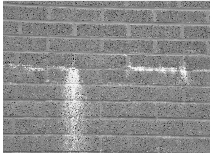
Figure 7 Deposits of calcium carbonate below a weep hole, as a result of the movement of water-soluble calcium hydroxide from the internal aggregate concrete blockwork being deposited over the brickwork
