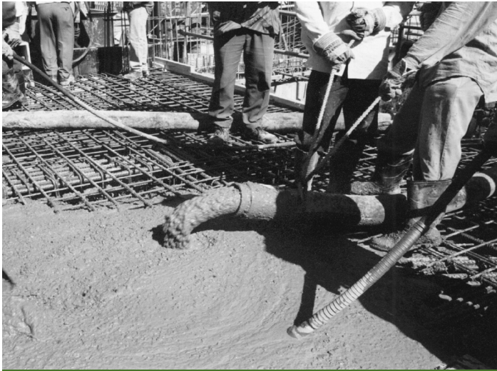
Figure 6 Superplasticised high-workability flowing concrete being used with dense reinforcement. Note that it is not quite self-levelling and a vibrator is still needed to ensure full compaction round the reinforcement
