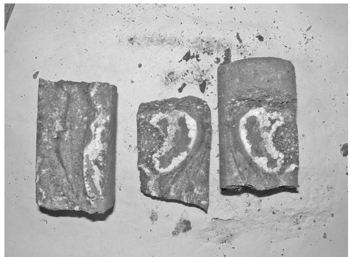
Figure 24 Masonry core of the railway bridge abutment shown in Figure 23. The blue-white crystalline deposit in the mortar joints is the reaction by-product thaumasite
