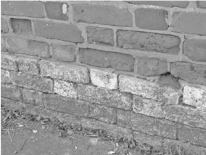
Figure 19 Salt fretting of an earth-retaining wall. The bricks below the ground level on the rear of the wall are heavily encrusted with calcium sulfate (gypsum) deposits, while above ground level the higher moisture content has resulted in frost damage
