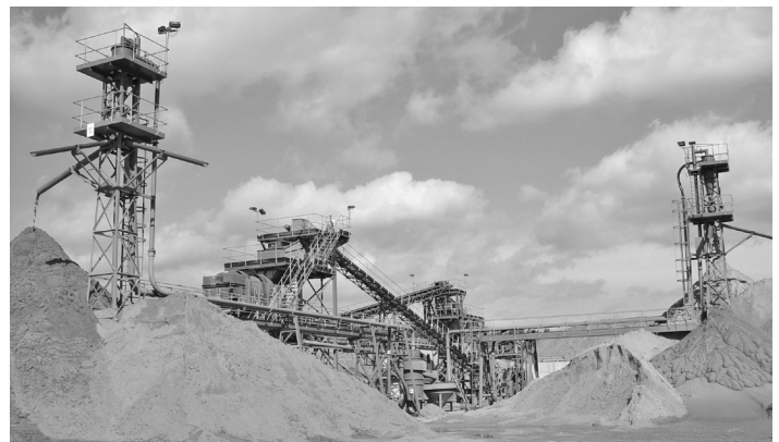
Figure 6 Sand and gravel plant (courtesy of QMJ Publishing Ltd)
