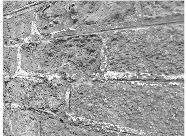
Figure 20 Example of gypsum (calcium sulfate) 'salt' crystal growth resulting in the 'blistering' of the brick face. Commonly seen on old earth-retaining walls and where infill behind walls, to allow drainage, are composed of furnace bottom ash and clinker/condensers. Both being naturally high in soluble sulfates
