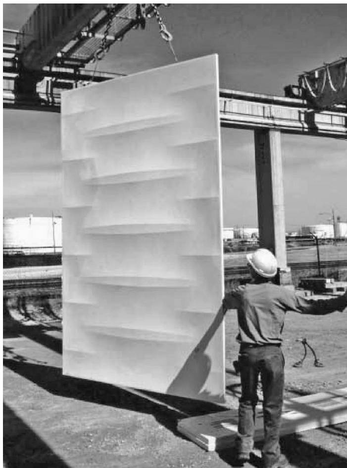
Figure 5 Precast wall panel produced using the fabric formed mould (M. West Fabric-formed concrete members, Concrete International, 2003)
