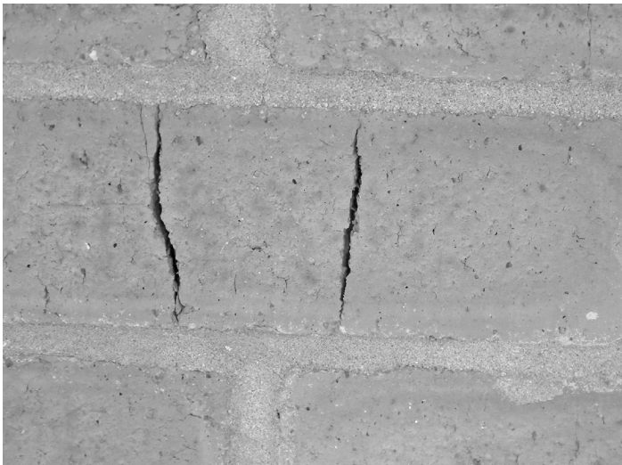
Figure 14 Fired cracks within bricks as a result of drying
