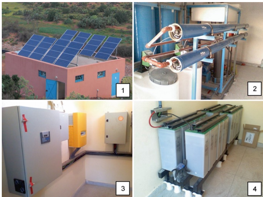
Fig. 22.9 Photos of the main components of an autonomous desalination system: 1. PV field on the roof of the building, 2. RO unit with the horizontal pressure vessels, 3. Control panel and electric converters, 4. Set of batteries
