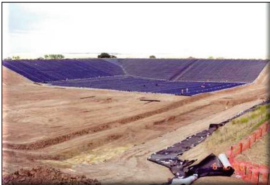
Fig. 4.8 Construction of the lining on-post hazardous waste landfill for contaminated soils. Source: US Army archives
