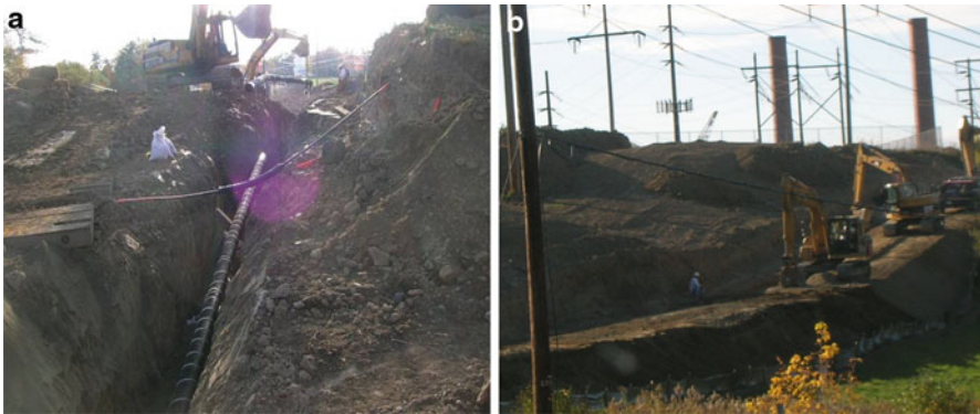
Fig. 12.1 Heavy machinery and soil disturbance during pipeline project right of way construction. Photo a Pipe installation in trench bottom across fallow land use type. Note vehicle traffic directly on top of subsoil spoil. Photo b Stripped topsoil segregated upslope from pipe in agricultural land use area. Vehicles shown backfilling subsoil spoil before topsoil
