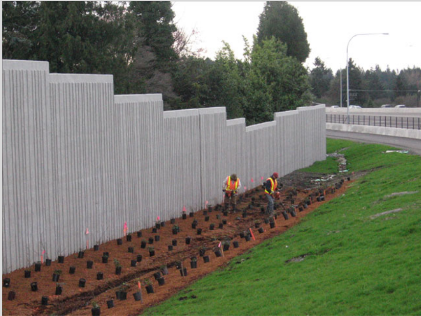
Fig. 9.7 Installing an experiment to test plant response to compost amendments along a highway right of way outside of Tacoma, WA (Data from this study is shown in Table 9.5. Photo credit: Andy Bary)
