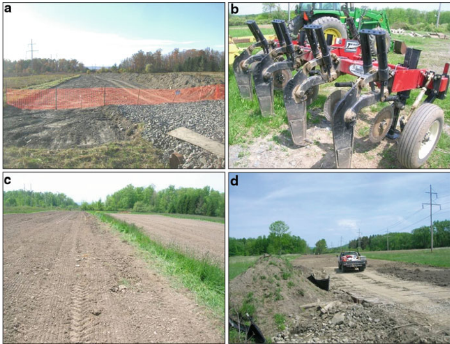
Fig. 12.3 Representative photos after pipe installation from pipeline project right of way. Photo a Agricultural land after pipe burial. Fall, 2008. Topsoil stockpiled on right . Photo b Unverferth zone-till ripper used to decompact ROW in agricultural land areas. Photo c Agricultural land (see Photo a ) after to drilling of grass mix. Spring, 2009. Photo d Wooden timber mats across ROW protect wetland soils. Soil berms and silt curtains control erosion
