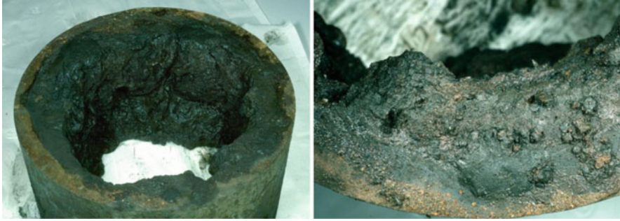
Fig. 3 Ochrous depositions in a drinking water pipe made from cast iron (diameter 25 cm), which had been in use for more than 80 years in Berlin, Germany
