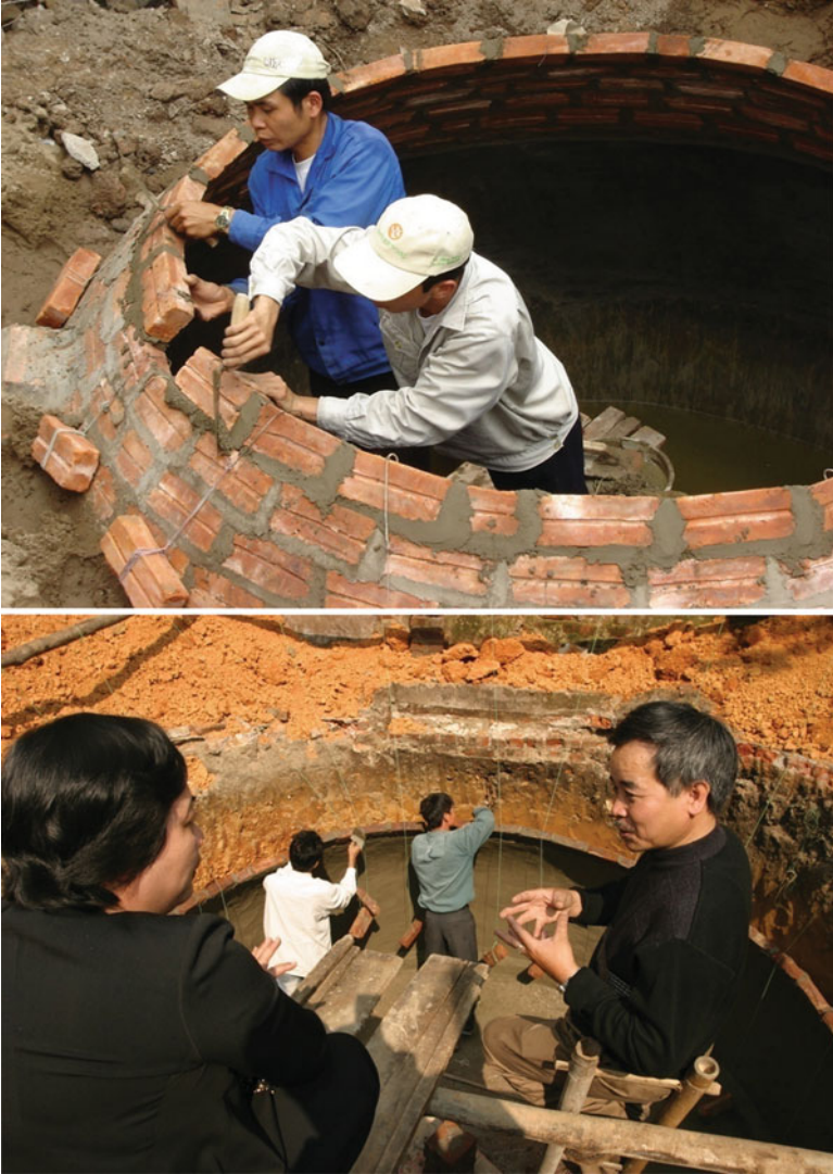
Fig. 2.3 Biogas plants being put up in Vietnam (photo courtesy: SNV, Netherland Development Organization)
