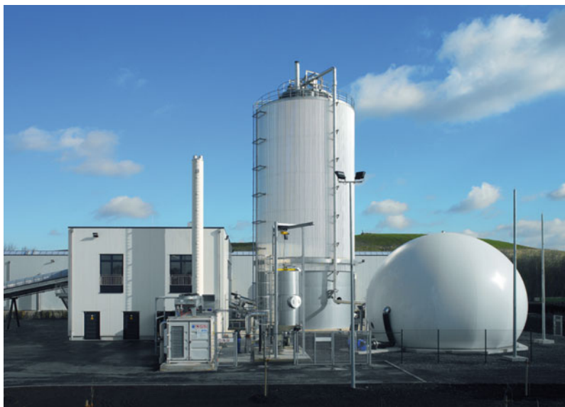
Fig. 7.16 A DRANCO plant at Münster (Germany) which treats 24,000 tonnes per year, of MSW (photo courtesy: Organic waste systems n.v.)
