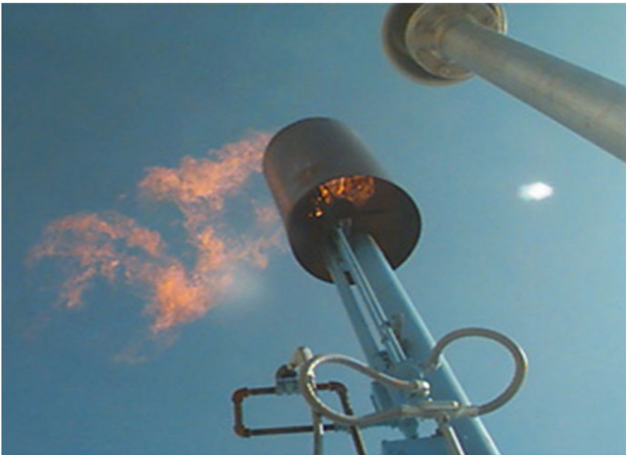
Fig. 5.20 Biogas being flared off (Photo courtesy: AgSTAR)
