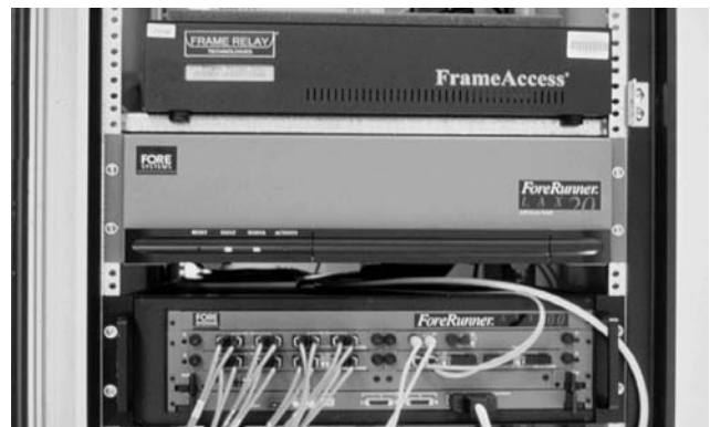
Figure 14. Example network switches and routers.
