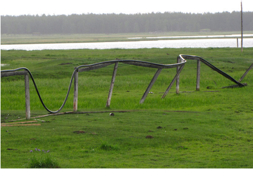
Fig. 4.7 Failed project: water pipeline in Uolba (Photo: Anna Stammler-Gossmann)
