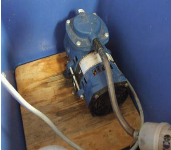
Fig. 9.3 Pump fitted to the overflow vessel
