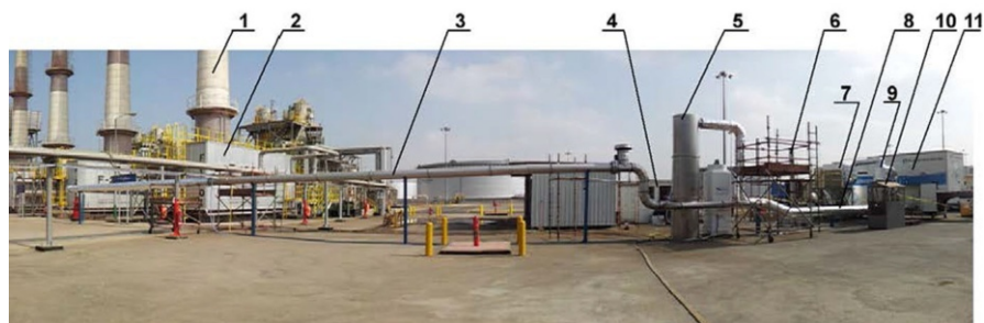
Fig. 7 General view of the pilot plant at Jeddah Refinery. 1 stack of F 1001 boiler, 2 boiler F 1001, 3 flue gas duct, 4 control room of pilot plant, 5 gas conditioning column, 6 pilot plant stack, 7 cartridge bag filter, 8 thermal insulated duct, 9 cyclone, 10 ammonia dosing unit, 11 mobile accelerator unit
