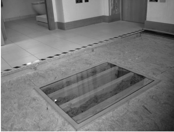
Figure 5.1 Insulation display, Sigma Ecohouse II, BRE Innovation Park, Watford, July 2007
