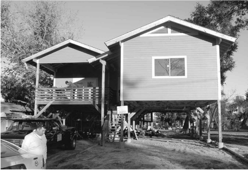
Figure 3.1 Architecture for Humanity project manager Michael Grote at the Nguyen house when it was under construction in Biloxi, Mississippi. Volunteers built homes high above potential future floodwaters using new wind-resisting tactics. Credit: James S. Russell
