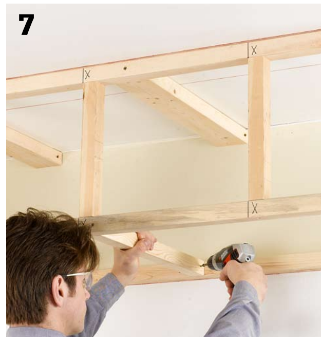
7 Cut crossmembers to fit between the bottom of the framework and the wall cleat. Attach the crossmembers by toe-screwing into the cleat and end screwing through the framework side. Place the crossmembers every 16" on center.
