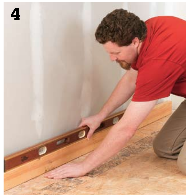
4 Find the highest point along the floor that will be covered by base cabinets. Place a level on a long, straight 2 × 4, and move the board across the floor to determine if the floor is uneven. Mark the wall at the high point.
