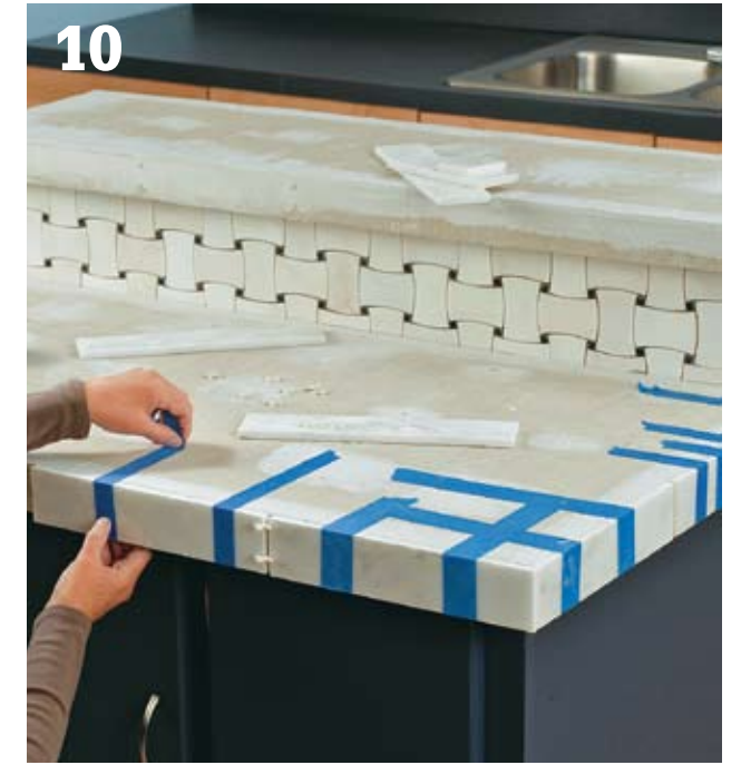
10 Cut the edge tiles and fasten them around the perimeter of the subbase with thinset adhesive. The tiles should be flush or slightly below the bottoms of the buildup strips and project past the top surfaces so they will be level with the field tiles. If you are not using edge tiles with a bullnose top, install the tiles so they are level with the subbase surface and overhang them with the field tiles.
