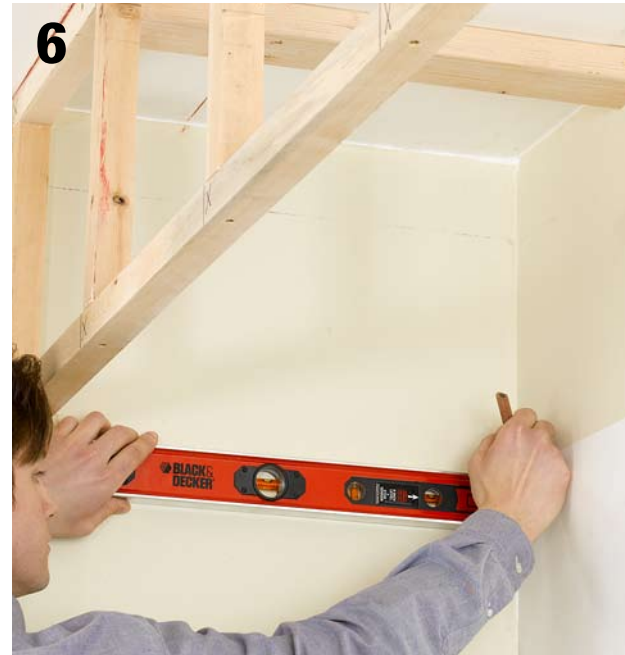
6 Use a level or laser level to mark the wall even with the bottom of the installed soffit framework. Cut 2 × 2s to the length of the soffit and attach this cleat to the wall aligned with the mark.
