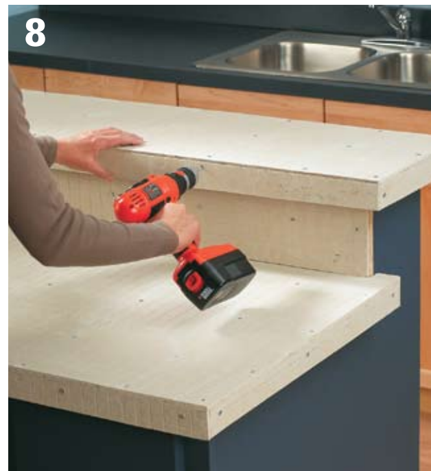
8 Attach the tile backboard to the counter subbases, the backsplash, and tape seams; cover screw heads with compound (see page 114).
