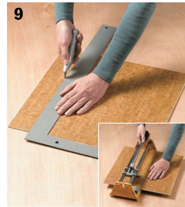
9 Cut the tile to fit using a utility knife and straightedge. Hold the straightedge securely against the cutting line to ensure a straight cut. Option: You can use a ceramic-tile cutter to make straight cuts in thick vinyl tiles (see inset).
