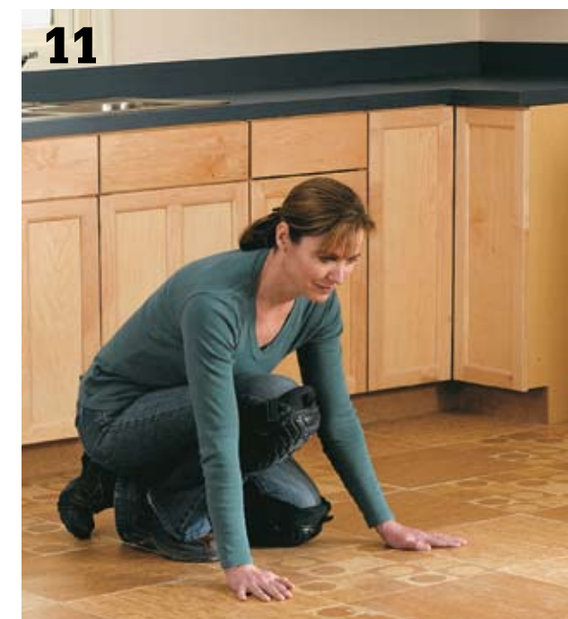
11 Continue installing the tile in the remaining quadrants until the room is completely covered. Check the entire floor. If you find loose areas, press down on the tiles to bond them to the underlayment. Install metal threshold bars at room borders where the new floor joins another floor covering.
