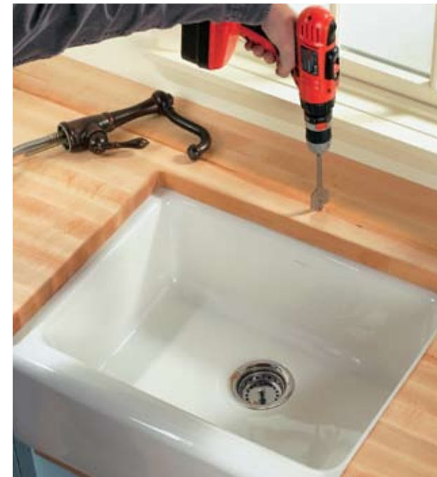
Option: If you're installing an undermount sink, mark a centerpoint for drilling a hole to accommodate the faucet body following the recommendations of the faucet manufacturer. A 1 3/8"-dia. hole is fairly standard.
