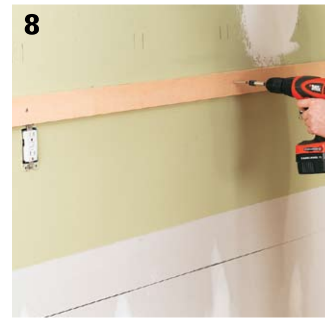
8 Install 1 × 3 temporary ledgers with top edges flush against the reference line lines. Attach ledgers with 2½" wallboard screws driven into every other wall stud. Mark stud locations on the ledgers. Cabinets will rest temporarily on ledgers during installation (the ledgers alone will not support them, however).
