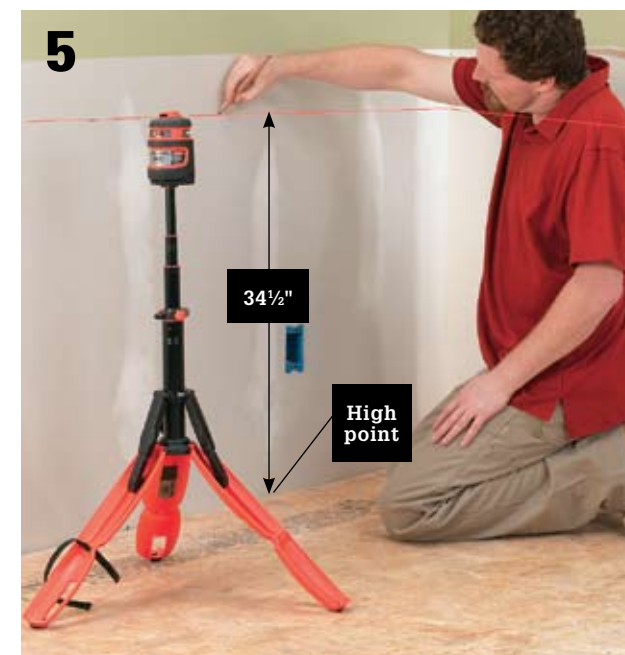
5 Measure up 34½" from the high-point mark (for standard cabinets). Use a level (a laser level is perfect) to mark a reference line on the walls. Base cabinets will be installed with top edges flush against this line.
