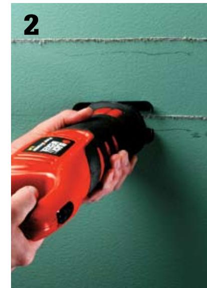
2 Plan the route for the new supply line beginning at the T-fitting and working toward the cooktop area. Determine the height of the new line and then snap chalklines from the sink to the cooktop. With the electrical power shut off, remove wall coverings 2" above and below the chalkline and at the location for the pot filler outlet. Make sure the location is high enough to clear your tallest stock pot.
