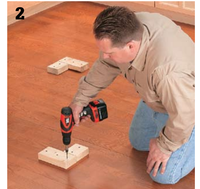
2 Cut 2 × 4 cleats to fit inside the inner outline to provide nailing surfaces for the cabinets. Attach the cleats to the floor with screws or nails. Tip: Create an L-shaped cleat for each inside corner.
