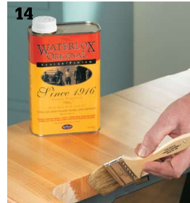
14 Seal the edges of the sink opening with a varnish as instructed by the butcher block manufacturer or by coating it generously with pure mineral oil or tung oil for a natural finish. Let sit for 15 minutes then wipe off the excess with a clean, lint-free cloth. Let it dry for 48 hours. Repeat six times, letting it dry thoroughly between coats.
