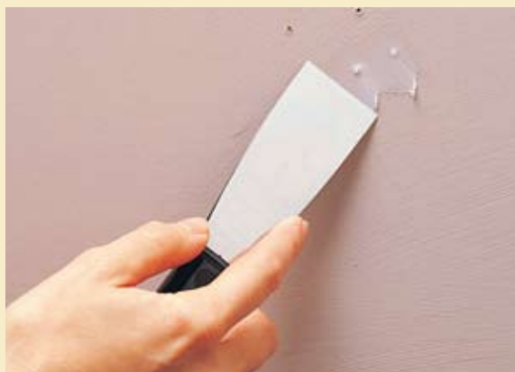
Apply lightweight spackle to holes with a putty knife or your fingertip. This keeps repair areas small. Let the spackle dry. Sand until smooth.
