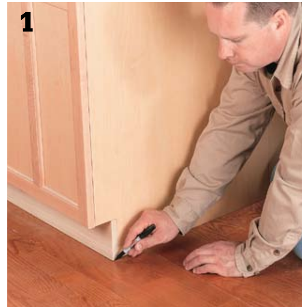
1 Set two base cabinets back-to-back in position on the floor and outline the cabinet corners onto the flooring. Remove the cabinets and draw a new outline inside of the one you just created to allow for the thickness of the cabinet sides (usually 3/4").
