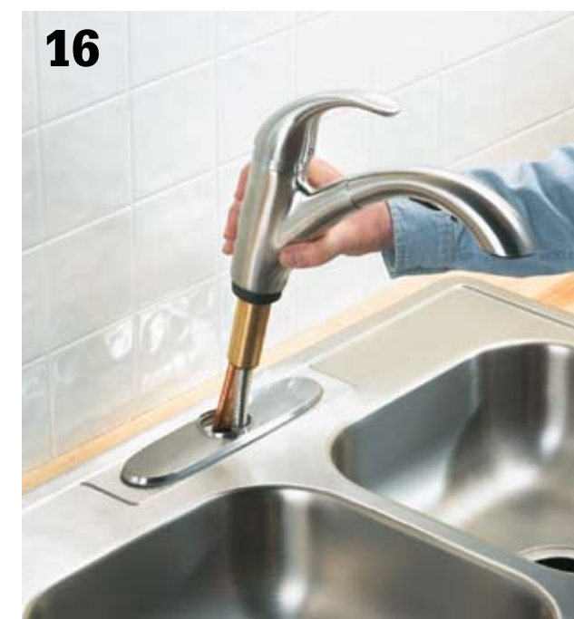
16 Install the faucet and sink and make the water supply and drain hookups (see pages 196 to 199).
