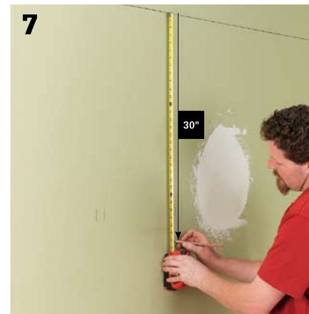
7 Measure down 30" from the wall-cabinet reference line and draw another level line where the bottoms of the cabinets will be. Temporary ledgers will be installed against this line.
