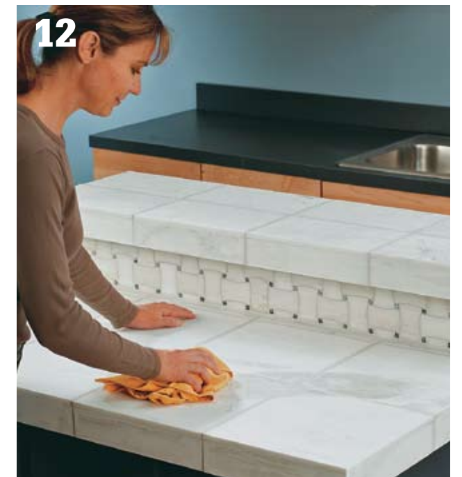
12 Choose a suitable grout color and apply it to the tile with a grout float. Buff off excess once it has dried. Seal the grout with grout sealer.
