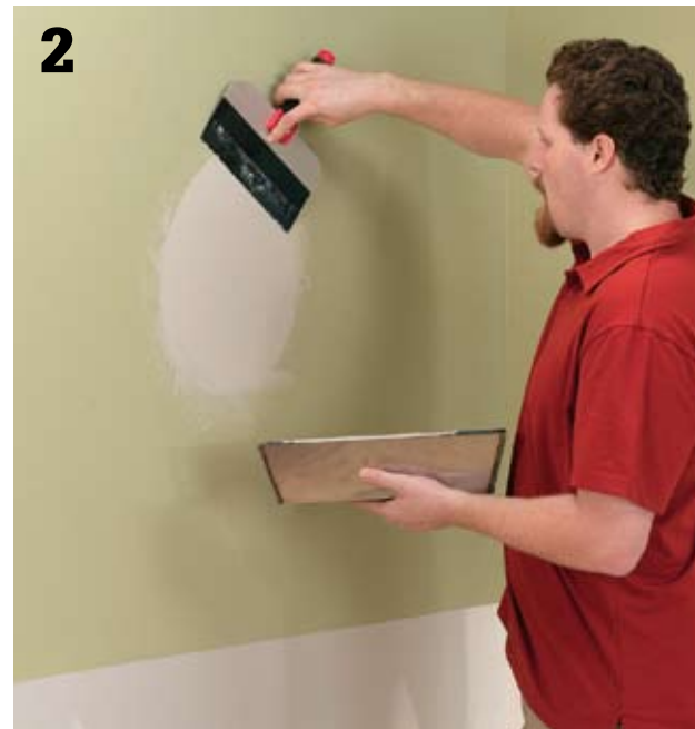
2 Fill in low spots in the wall by applying wallboard compound with a taping knife. Let the compound dry, and then sand it lightly.
