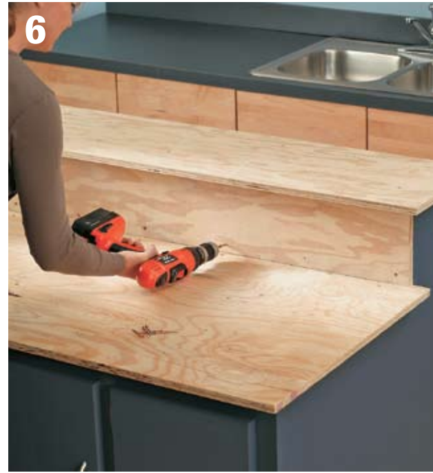
6 Cut strips of 3/4" exterior plywood to make the subbases for the countertops and a backer for the backsplash. The lower counter subbase should overhang by 2" on the front and sides. The upper should overhang 2" on the sides and be centered on the cabinet front to back. Attach the backer and subbases with drywall screws driven down into the 2 × 4 cross supports.
