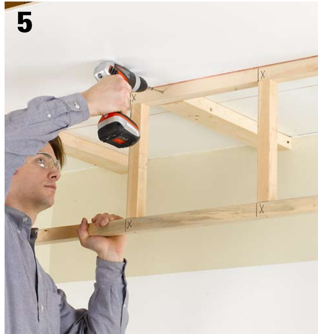
5 Attach the soffit framework to the ends of the 2 × 4s with drywall screws.
