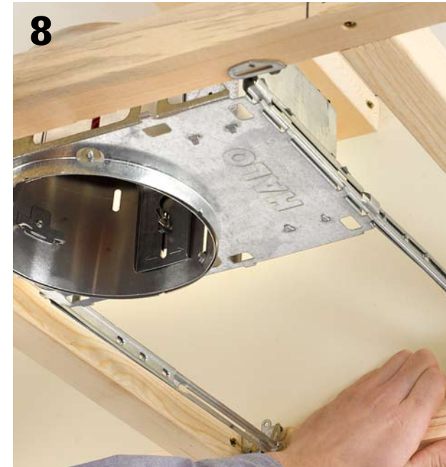
8 Install lighting or ductwork, if needed. Extend the mounting bars on recessed fixtures to reach framing members.
