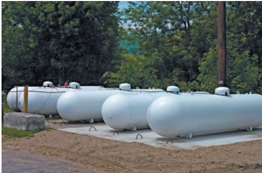
Photo 7.3 Cylindrical pressure vessels for liquid propane.
