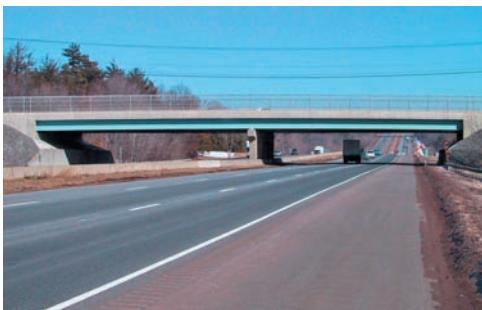
Photo 9.3 The continuous beams supporting this highway overpass have three supports and are thus statically indeterminate.
