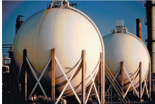
Photo 7.4 Spherical pressure vessels at a chemical plant.
