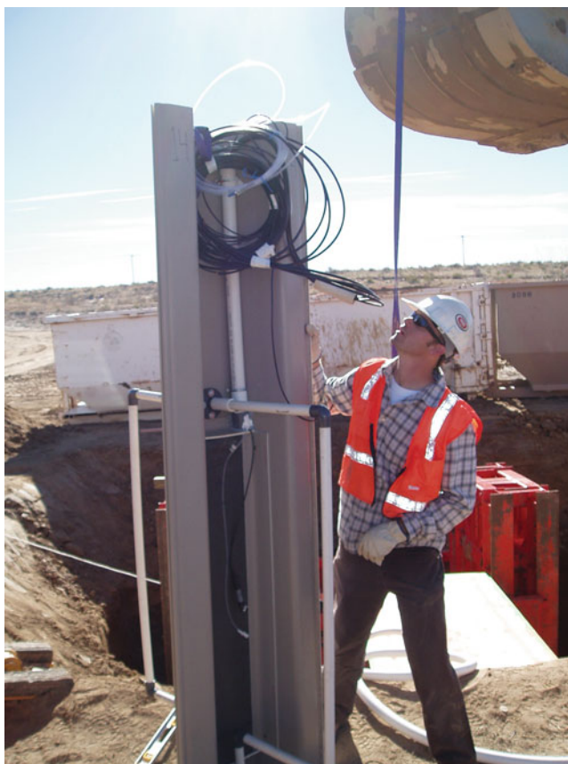
Figure 17.3. Individual electrode panel mounted to vinyl sheet pile sections forming a single e-barrier module. 15 e-barrier modules were installed at the Pueblo Chemical Depot for management of a groundwater plume containing energetic compounds.
