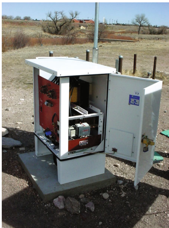
Figure 17.11. Rectifier used for power to the e-barrier (Corrpower, Inc., Chardon, Ohio) (from Sale et al., 2005).
