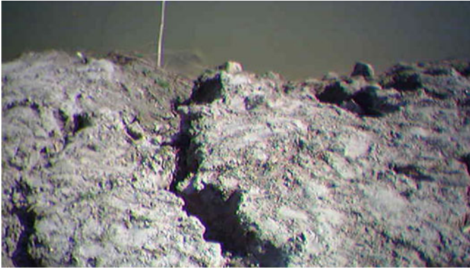
Fig. 17 Formation of a wide gully on the bare riverbank
