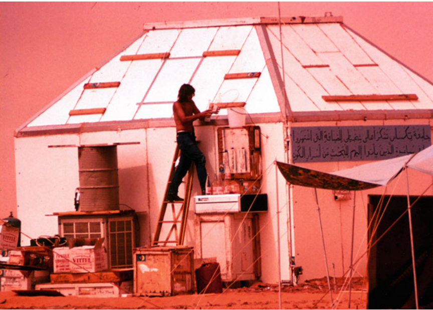
Fig. 6b Building the Observatory. Burton Jones sets up the refrigeration by cooling
