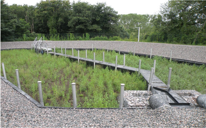
Fig. 6.7 The view of VFTW for combine sewer over flow in France near Lion ( Photo M. Gajewska )
