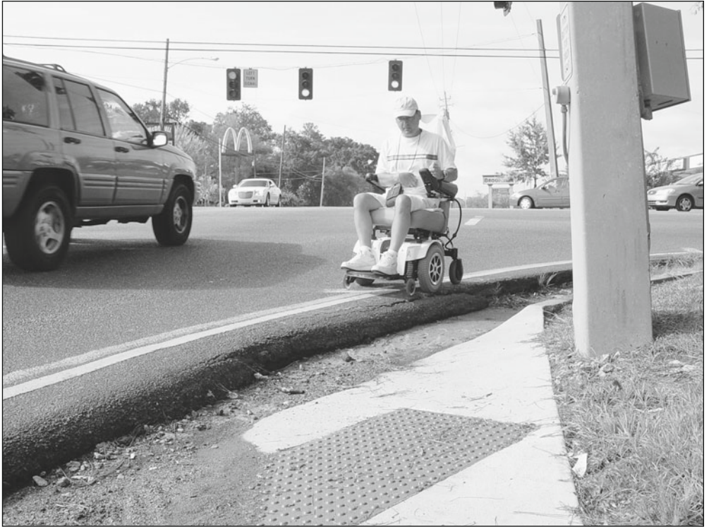
Complete streets policies should end disconnects like this one. (Photo by Judy McNeil.)
