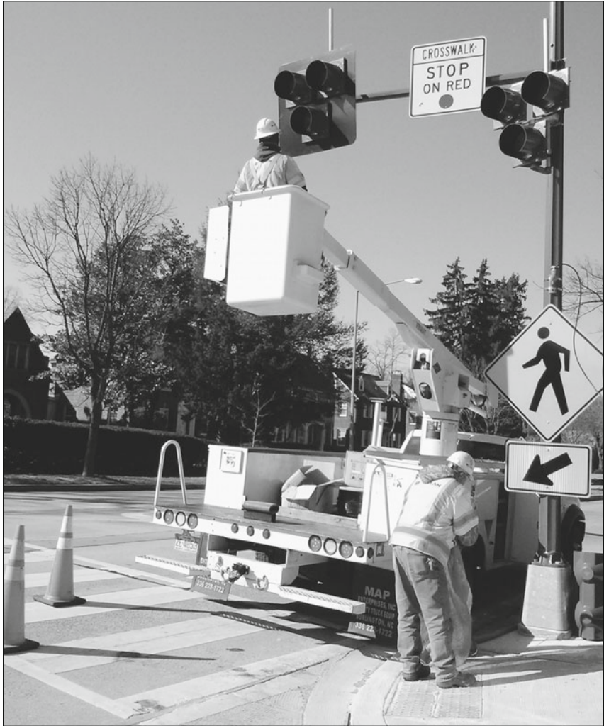
A crew in Washington, DC, installs a HAWK (high-intensity activated crosswalk) beacon on a busy arterial. These signals are now recommended by the FHWA as a safety countermeasure. (Photo by Barbara McCann.)
