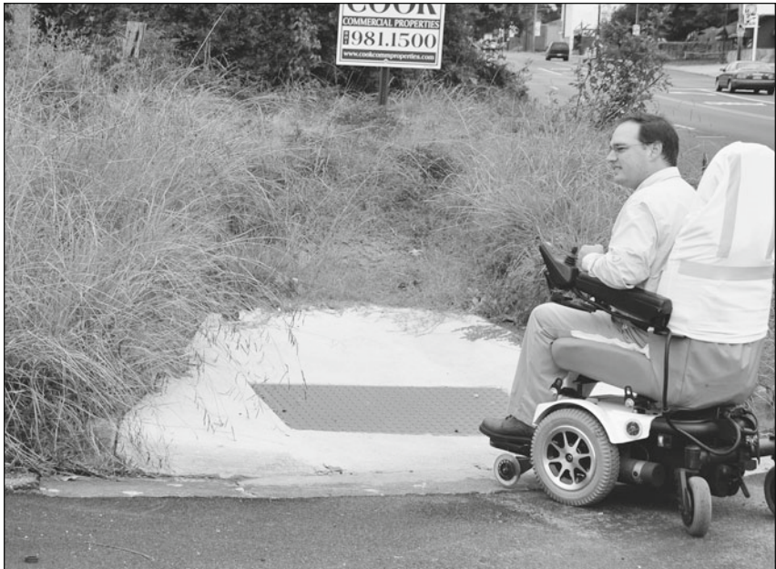
Curb ramp to nowhere in Jackson, Mississippi. (Photo by Judy McNeil.)
