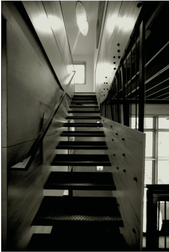
Figure 12.7 The wall veneers in this stairwell are made of durable fiberboard that ensures longevity. The metal steps are made of 50 percent recycled content steel, and the wood ceiling joists are all reclaimed.
