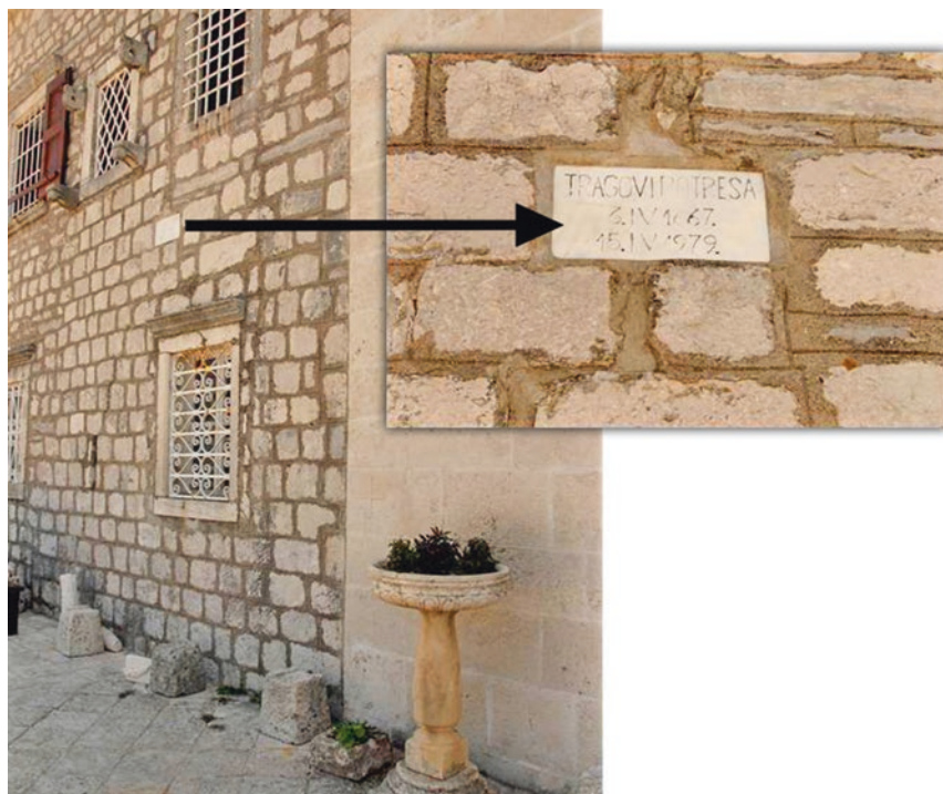
Fig. 3.14 Scoglieto della Madonna, wall of the monastery: a fissure running from top to bottom is highlighted by a sign, which says “Traces of the earthquakes of 6 April 1667 and 15 April 1979” (photo by PA, 2011)
