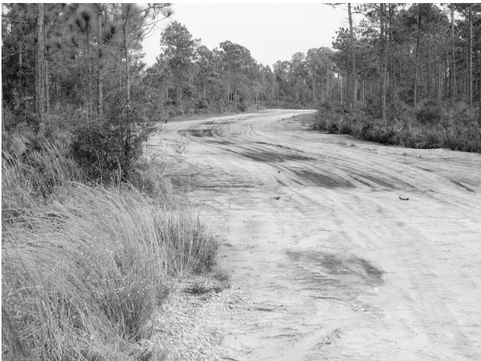
FIGURE 9.2. Forest road near the one shown in fig. 9.1 in which the side ditches were filled and the roadbed graded to restore hydrological processes.
