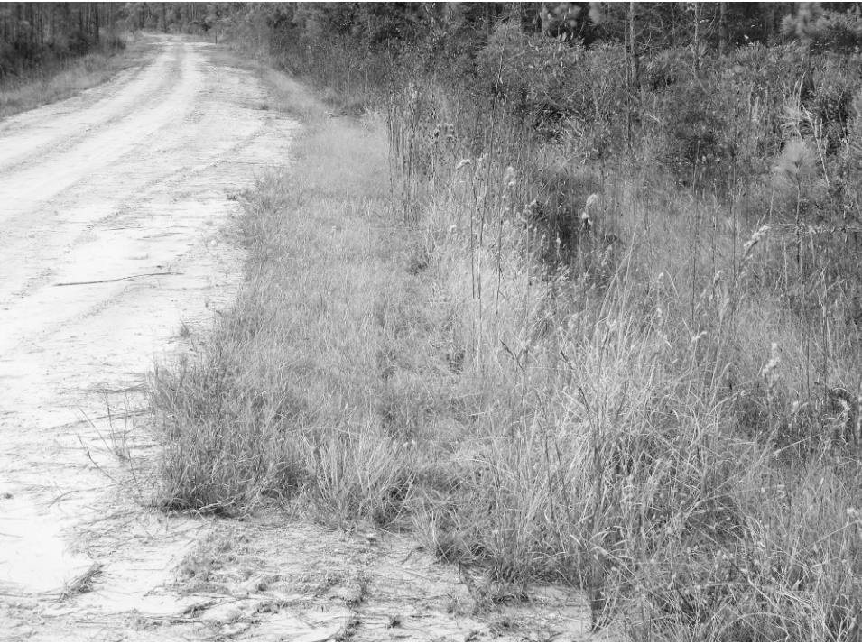
FIGURE 9.1. Typical graded forest road drained by a ditch on either side in Florida, USA. The ditch and slightly elevated road intercept surface runoff of precipitation and modify the hydrology in adjacent pine savanna.
