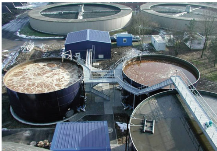
Fig. 6.1 SBR “Rosenheim”, Germany
