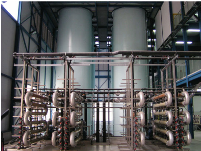
Fig. 6.5 Leachate treatment plant Bilbao, Spain, built by Wehrle Umwelt
