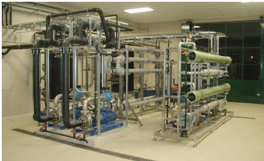
Fig. 6.11 Ultrafiltration and reverse osmosis units in a MBR+RO plant in a landfill of Girona, Spain, built by Wehrle Umwelt
