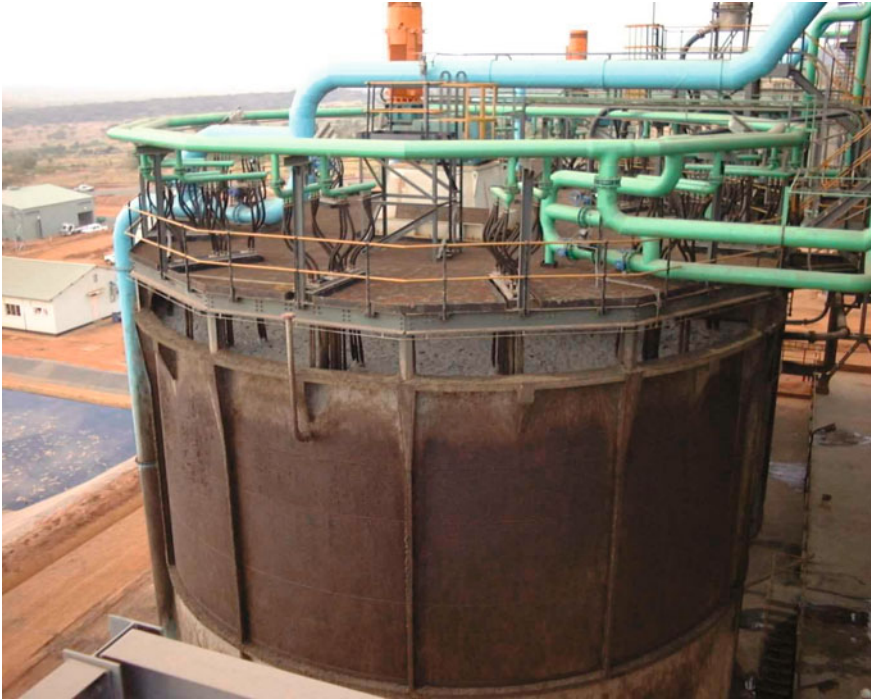
Fig. 3 Stirred-tank bioleaching plant at Kasese, Uganda (picture from BRGM/Kasese Cobalt Company Ltd.)
