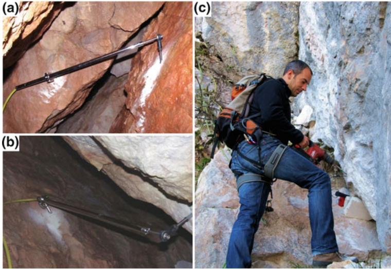
Fig. 4.6 Installation of the strain gauges: a strain gauge 3, installed in the middle of the failure cave; b strain gauge 4, installed at the end of the accessible area inside the failure cave; c Prof. Dr. Michael Krautblatter installing strain gauge 1 at the outside of the critical block
