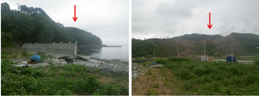
Fig. 4.3 Damaged seawalls and area for relocation in the mountain ( left ). Forests in the mountain that were cut for personal purposes ( right )
