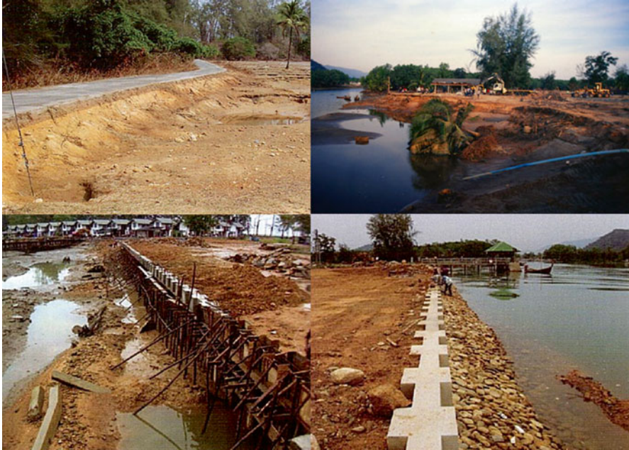
Fig. 6.12 Typical road damages ( top left ; early 2005) and erosion damage due to the tsunami wave along the Kamphuan canal ( top right ; December 2004); rebuilt of the Kamphuan canal's banks ( bottom ; mid 2005) behind the ACRSD (Source: ACRSD)
