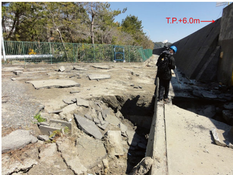
Fig. 13.11 Intact parapet and broken apron concrete with land scoured by overflowed tsunami in Power Plant District (March 25, 2011). The location is marked in Figs. 13.8 and 13.14
