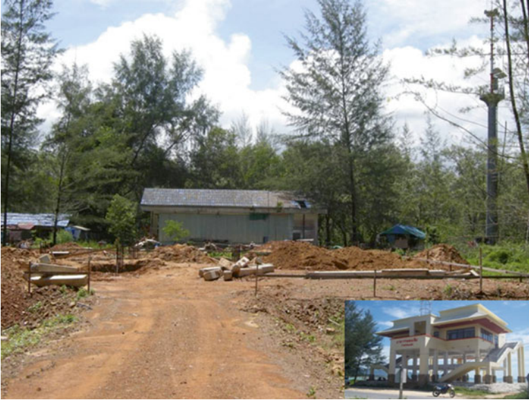
Fig. 6.16 The construction site of the standard emergency tsunami shelter (inset) at the Nua village, Kamphuan subdistrict, Suk Samran district, Ranong province that is funded by the government
