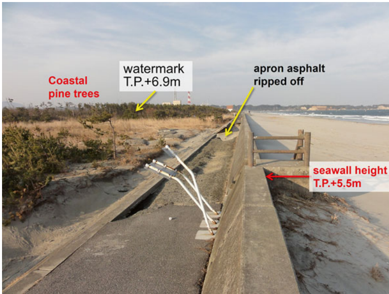
Fig. 13.16 Partially broken seawall and coastal pine trees in Suga District. The photograph was taken at the seawall on the line ‘S1’ marked in Fig. 13.8 (April 1, 2011). The watermark in the pine trees is the most seaward measurement plotted in Fig. 13.15b
