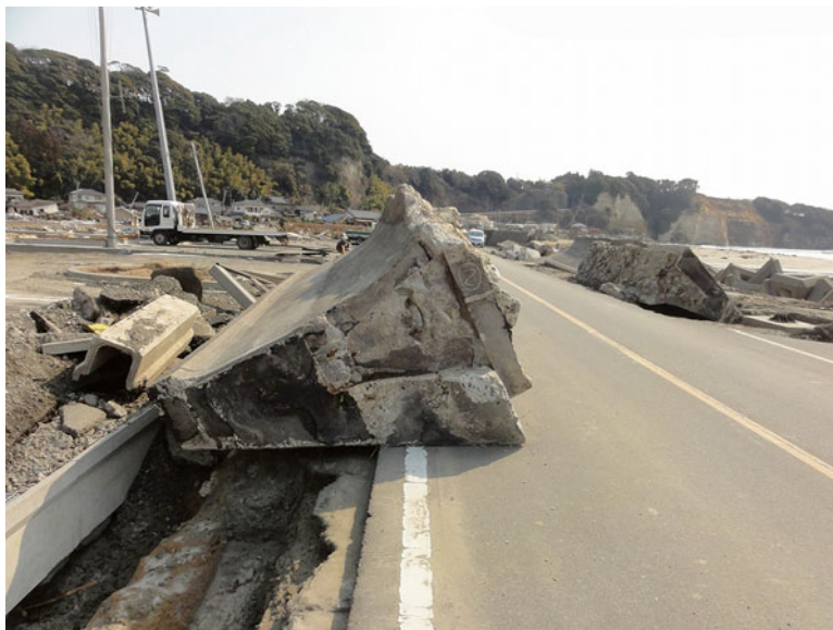
Fig. 13.13 Displaced and Broken seawall block in Iwama District (March 25, 2011). The location is marked in Figs. 13.8 and 13.14
