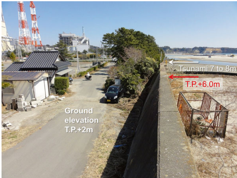
Fig. 13.10 Insignificant damage behind a high seawall in Ooshima District. (March 25, 2011). The location is marked in Figs. 13.8 and 13.14
