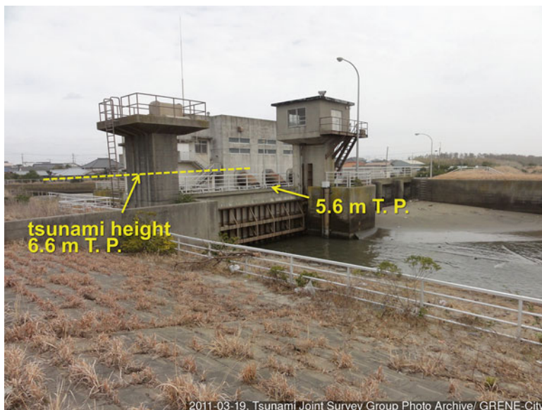
Fig. 13.6 Water gate at the Shimbori River mouth, Chiba Prefecture (March 19, 2011); measured watermark height was 6.6 m T. P. and 1.0 m higher than the top of the gate (UTMS-0163 in the TTSG database, location marked in Fig. 13.2)
