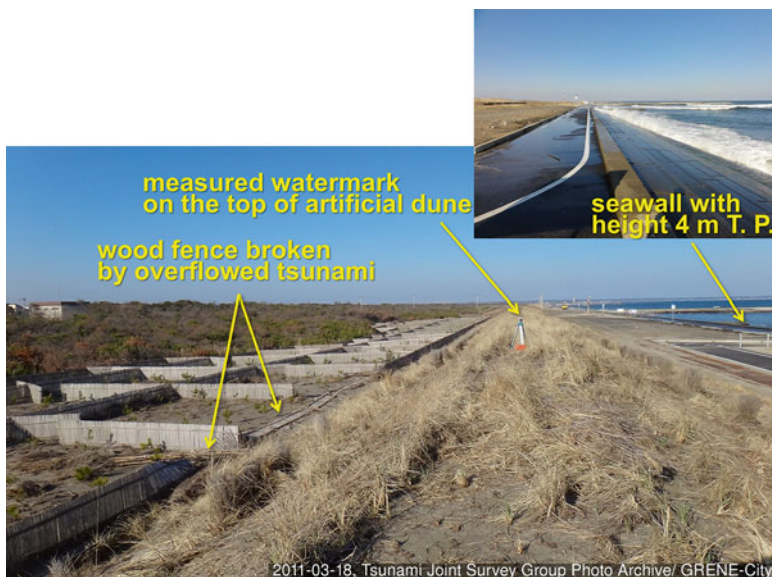
Fig. 13.5 Tsunami watermark measured on Kujuukuri Beach, Chiba Prefecture (March 18, 2011); a watermark was measured on the top of an artificial dune, 6.2 m T. P. and 17 m from the shoreline protected by a seawall with height 4 m T.P. (UTMS-0209 in the TTSG database, location marked in Fig. 13.2)
