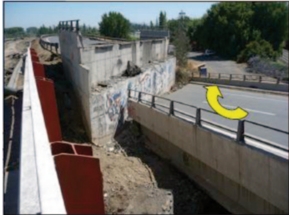
Fig. 26 Collapse of hospital overpass
