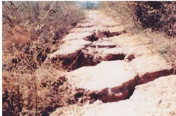
Fig. 10 Tapar dam Transverse crack on the crest. (after Yadav et al. 2008)
