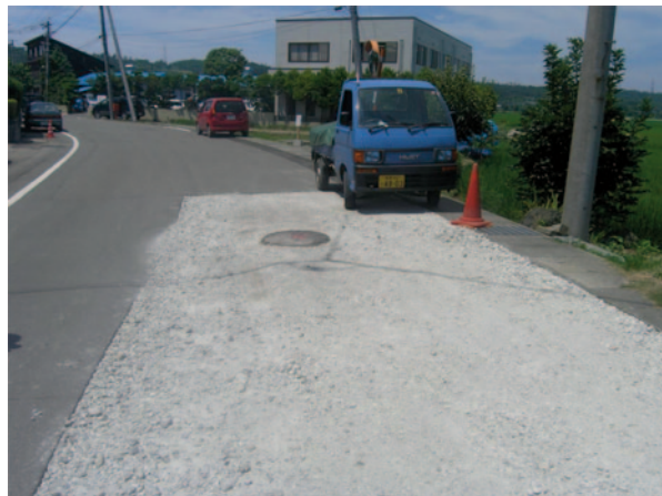
Fig. 2 Prevention of liquefaction damage of lifeline by backfilling by using cement-mixed soil
