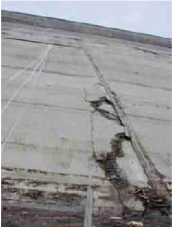
Fig. 25 Zipingpu dam joint damages. (after Chen 2008)
