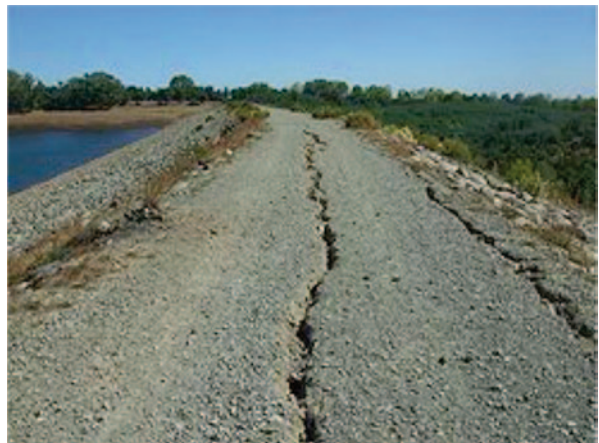
Fig. 14 Coihueco Dam -Longitudinal cracks at the crest
