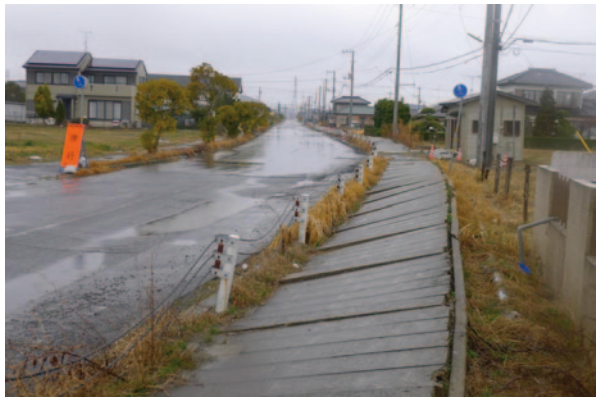
Fig. 16 Outward distortion of the box-type buried drainage channel installed along the roadside at the site A in Fig. 13—A view to the northeast
