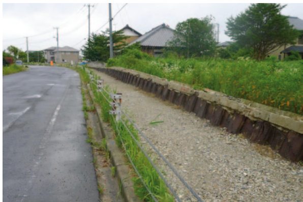
Fig. 17 Lift up and outward distortion of the buried sheat pile row accompanied by lateral displacement at location B in Fig. 13—A view to the eastsouth
