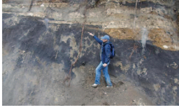
Fig. 30 View of Fujinuma Dam Embankment fill layers on top of black organic foundation residual soil exposed within downstream slope at left abutment
