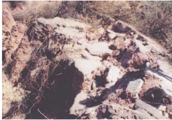
Fig. 9 Tapar dam Failed Maximum Height channel section. (after Yadav et al. 2008)
