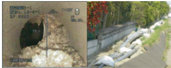
Fig. 1 Clogging and floating of sewage pipes. (From website of Urayasu City)
