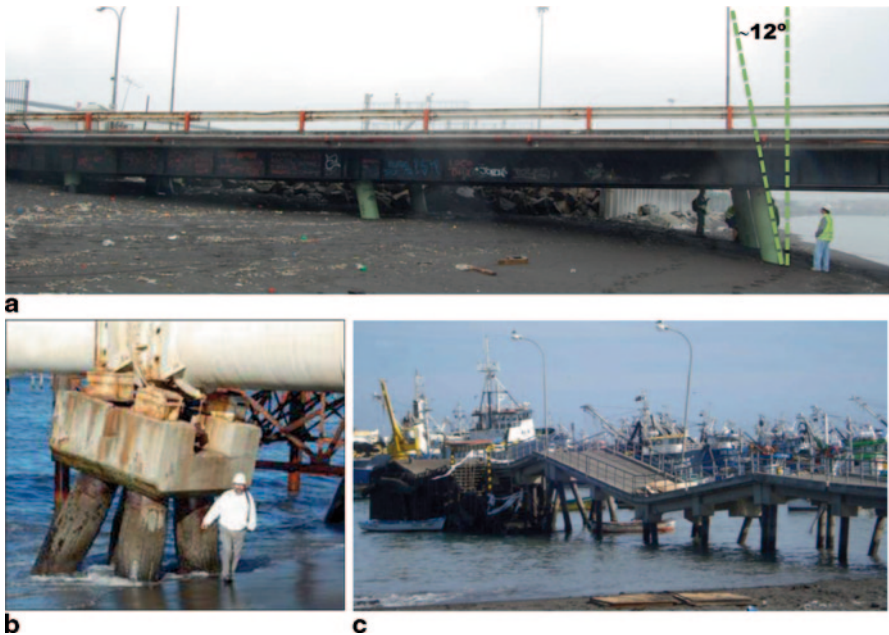
Fig. 17 Lateral spreading. a Coronel Port. b Bocamina Port and. c fishermen's Port of Coronel
