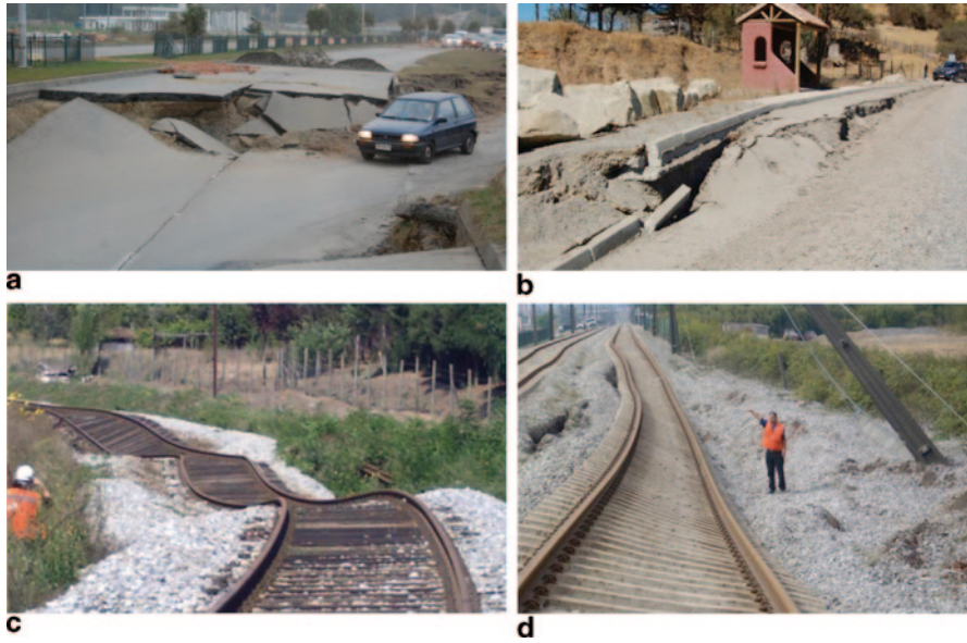
Fig. 11 Post-liquefaction settlements. a Costanera route in Concepción. b South access to Yali bridge near Navidad. c and d Railway near Concepción
