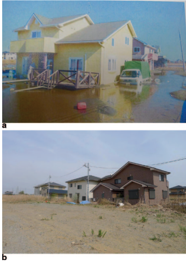
Fig. 35 Sinking and tilting of houses in the Fukashiba district of Kamisu. a Mud water around private houses. b Private houses tilted and subsided
