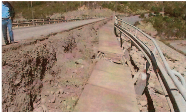
Fig. 16 Colbun earth Dam with 2 m horizontal displacements and 1 m vertical displacements
