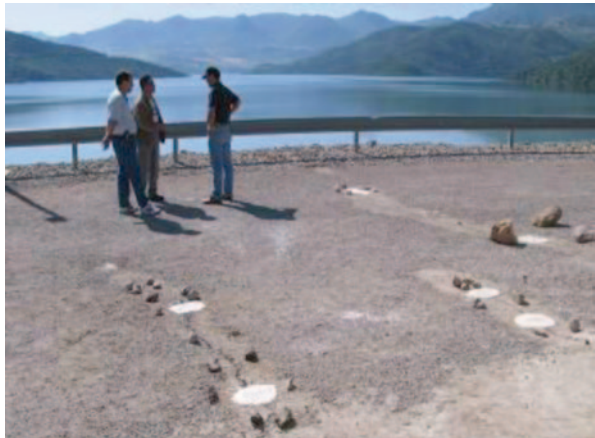
Fig. 22 Keddara dam-cracks observed at the crest
