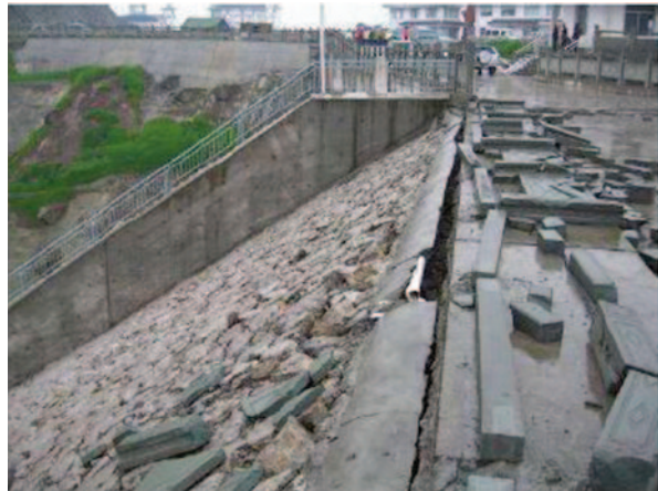
Fig. 24 Zipingpu dam crest damages. (after Chen 2008)
