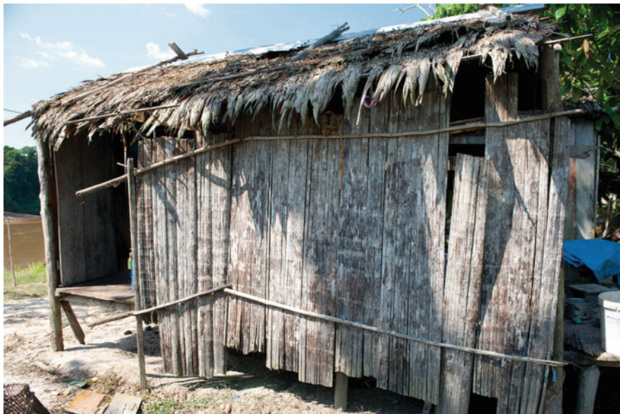
Fig. 40.3 Wall of an external kitchen fashioned with the split stems of paxiubinha. The roof is thatched with fronds of caraná ( Mauritia carana ) palm. Cacaububa, Tefé River, Amazonas, Brazil, 9-10-12
