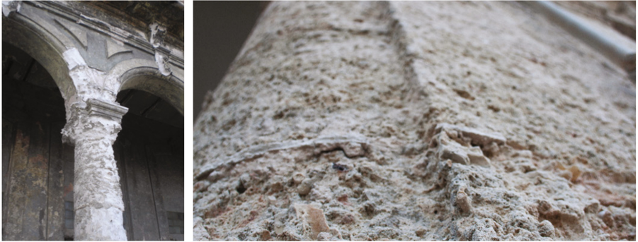
Fig. 2. Building Malecon 21. Stone column covered by highly porous lime mortar, intensely disintegrated on the surface, likely due to salt crystallization. Buildings have had no restoration intervention since 1910.
