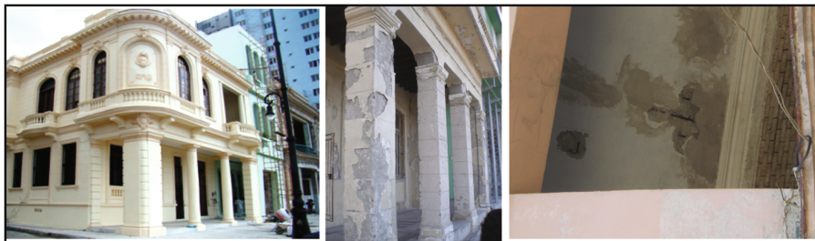
Fig. 1. Building Malecon 251 (left) Main substrates of brick masonry and reinforced concrete. Restoration work: waterproofing of roof, repair of renders on the facade and columns. Repair of renders was done with MAXREST and lime-based mortar. (center, right)
