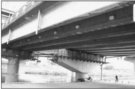
Figure 6. The monitoring system of Kia Bridge.
