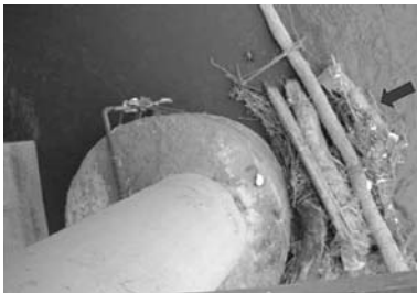
Figure 5. Floating debris accumulation at upstream of UP12 in the flood.
