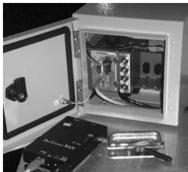
Figure 1. Prototype of structural monitoring system adopting automation technology.
