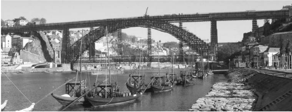
Figure 1. Overall view of Luiz I bridge during the ongoing strengthening and rehabilitation works.
