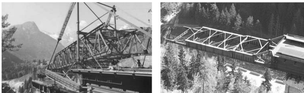
Verrand viaduct. Lattice girders (launching from Aosta yard and from Monte Bianco yard)
