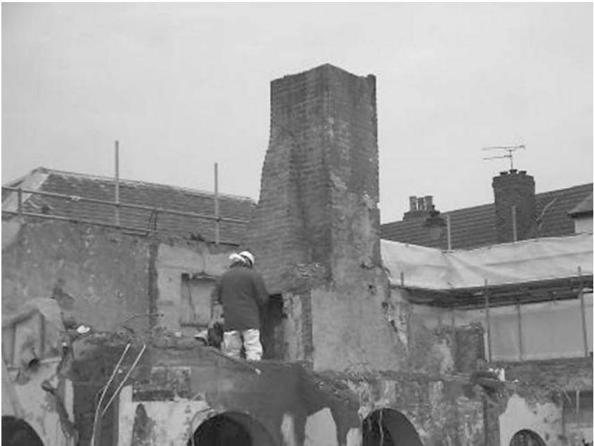
Figure 8.3 Demolition of the fireplace and chimney flue, alongside which much of the Sittingbourne Cache was discovered. Image Credit: Textile Conservation Foundation
