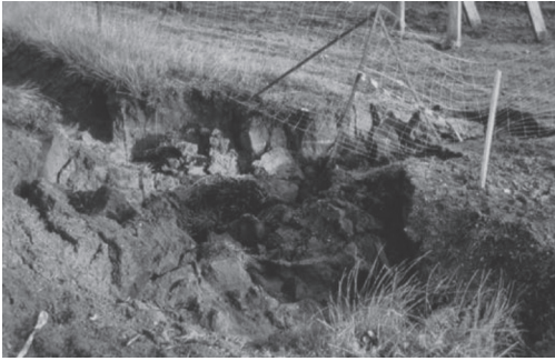
Figure 2. Collapse behaviour in shallow layers of loess directly exposed to climatic variations.
