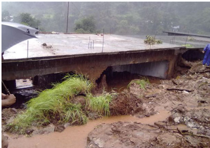
Fig. 12.9 A view of Primary School hit by landslide where 18 children were buried alive
