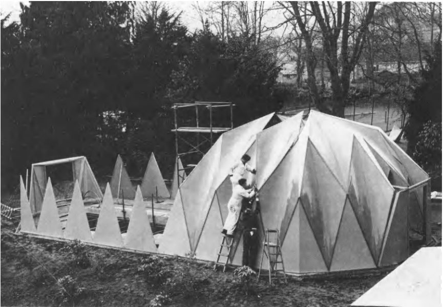
Figure 8.2 Swimming pool enclosure made up of GRP hyperbolic paraboloid modules to form a ‘folded plate’ structure
