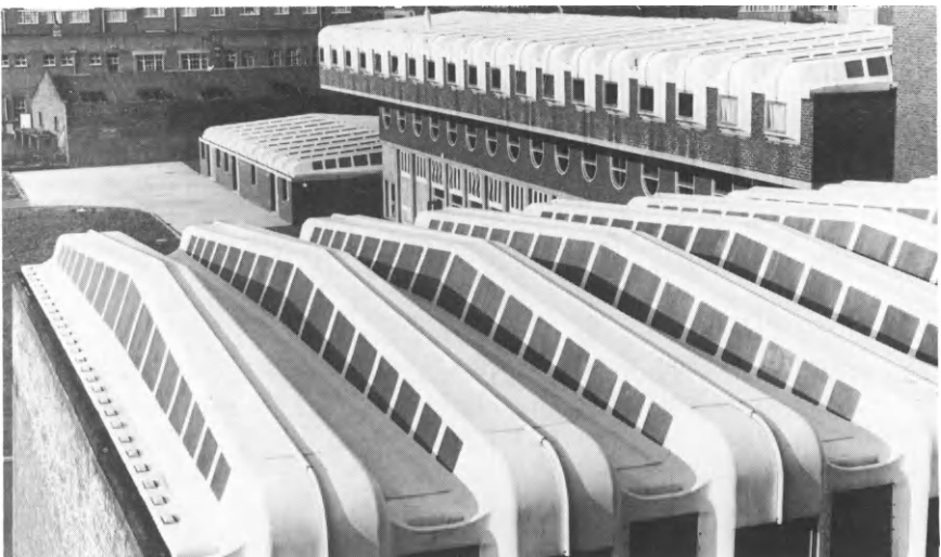
Figure 10.3 GRP roof for school in Stepney, London. Note joints at ridge of troughed sections and translucent panels
