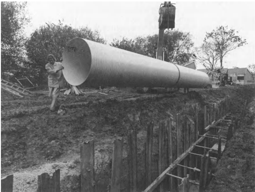
Figure 5.13 Large diameter GRP pipe
