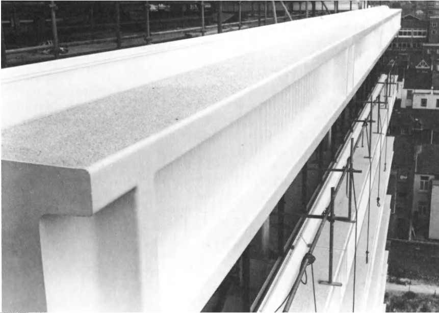
Figure 3.1 GRP detail from American Express building, Brighton. Although there is a strong influence here of pre-cast concrete, the geometric precision, colour and texture, could be obtained only with GRP. Note the moulded-in non-slip walking surface for window-cleaners
