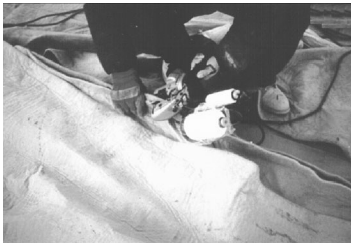
Figure 7-6. Sewing of a Geotextile Field Seam in a "Flat" or "Prayer" Seam Type.
