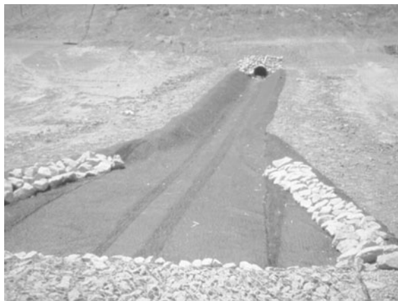
(c) Stone-filled gabions as a PERM (hard armor).
