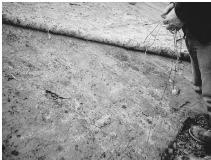
(b) Fugitive bentonite resulting from extrusion of hydrated bentonite through woven geotextile of GCL
