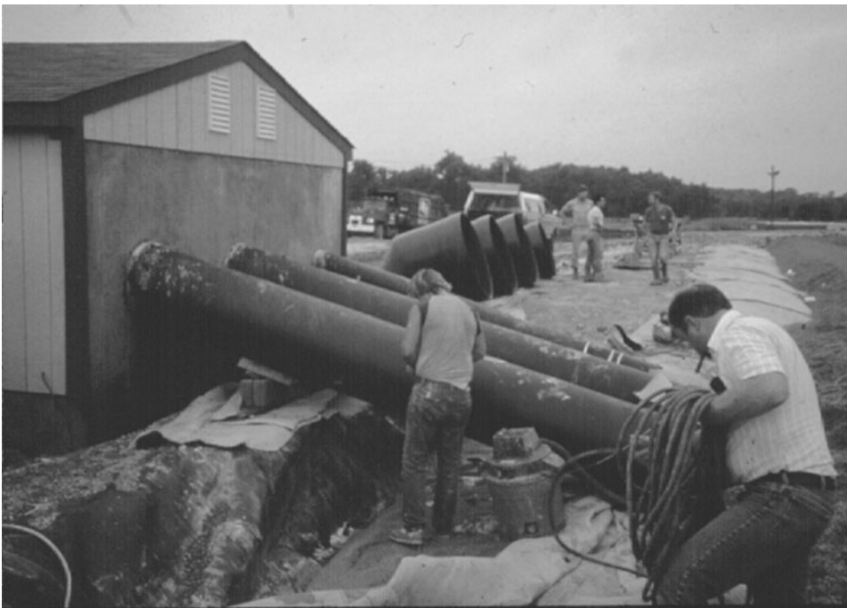
Figure 9-4. HDPE Smooth-Wall Pipe Risers Used as Primary (Two Redundant Pipes) and Secondary (in Background) Removal Systems Extending from Sump Area to Removal Shed.
