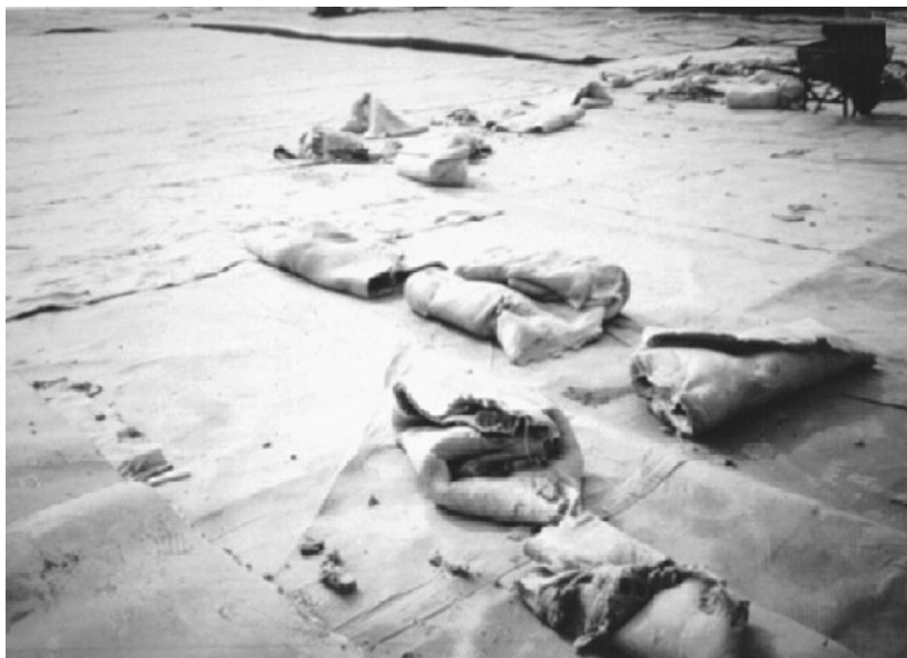
(a) Premature hydration of a geosynthetic clay liner being gathered and discarded because of its exposure to rainfall before covering
