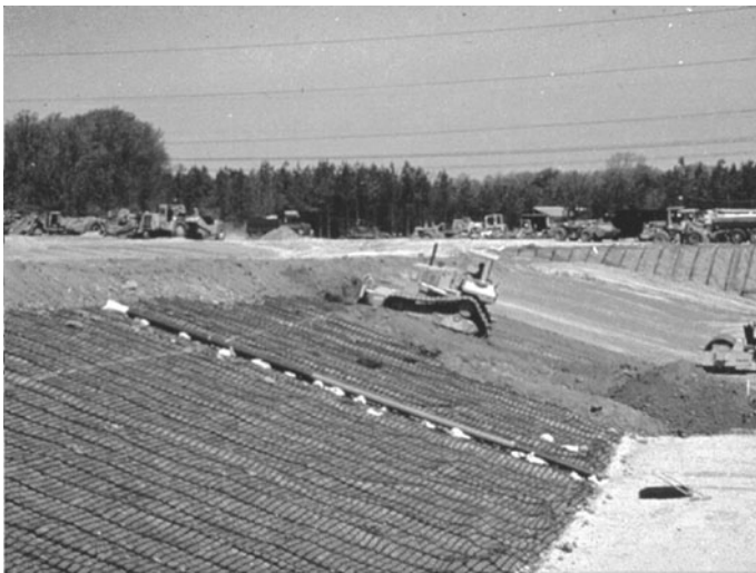
(b) Geogrids used as veneer reinforcement. Note that backfilling is proceeding from the bottom to the top of the slope.
