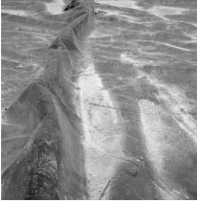
Figure 4-16. Excessively Large HDPE Geomembrane Wrinkle.
