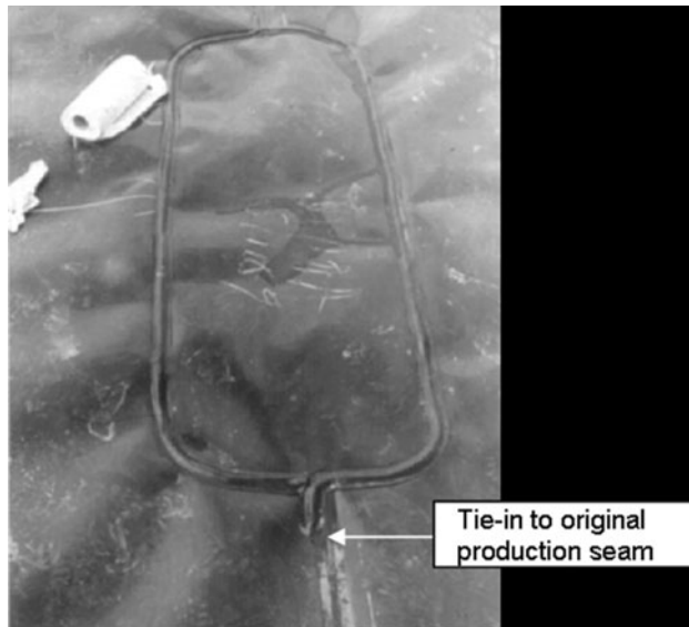
Figure 4-23. Completed Patch on a Geomembrane Seam That Had Previously Been Sampled for Destructive Tests.
