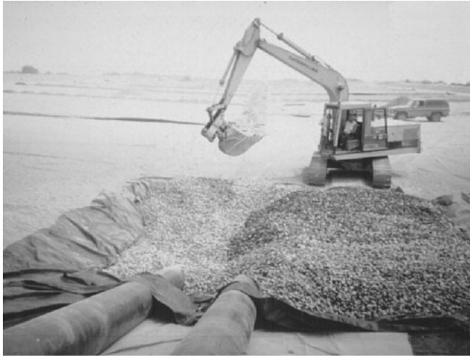
(a) A shallow sump area with redundant leachate removal pipes
