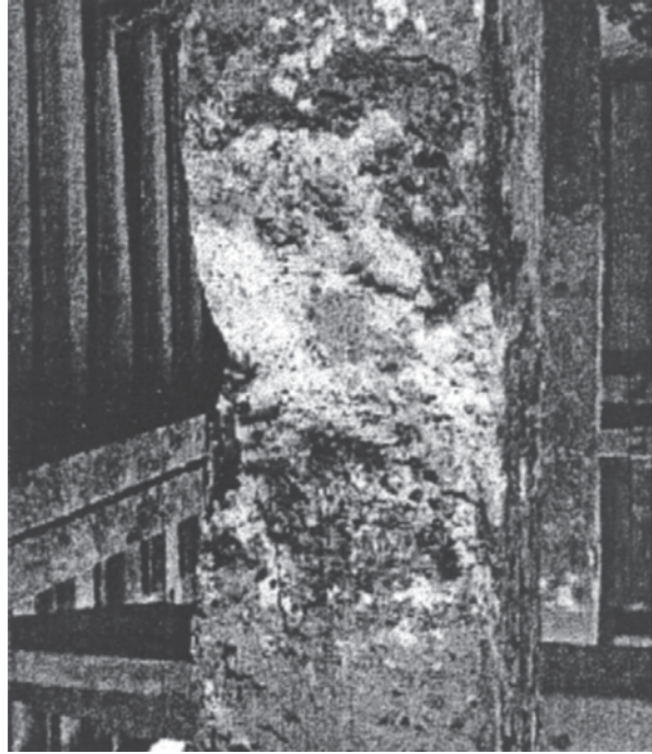
Fig. 6.67 Thaumasite sulphate attack in a structural beam—the bridge support in the motorway (Photo courtesy of Halcrow Group Ltd, U.K.). (According to [273])
