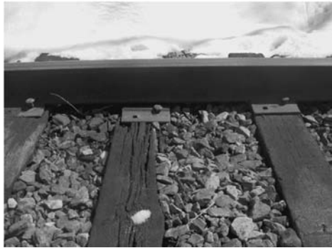
Figure 1: Deteriorated wood ties and loose rail spikes after seven years.
