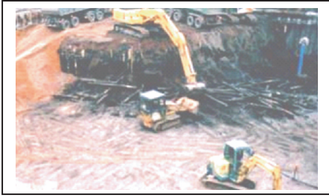
Figure 3. Thousands of wooden piles are excavated while creating a new underground development in Hamburg, Germany.
