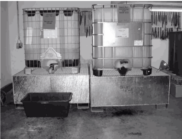
Figure 5. Retention trays for containers with a volume of 1000 l. The tap at the left container is protected by an additional tray to retain small leakages from filling procedures. The whole storage room is constructed as a retention basin and coated with a chemical-proofed coating.
