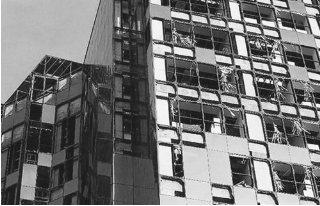
Figure 9. Other office buildings were severely damaged by hurricane Wilma. (Courtesy of Steven Camposano).
