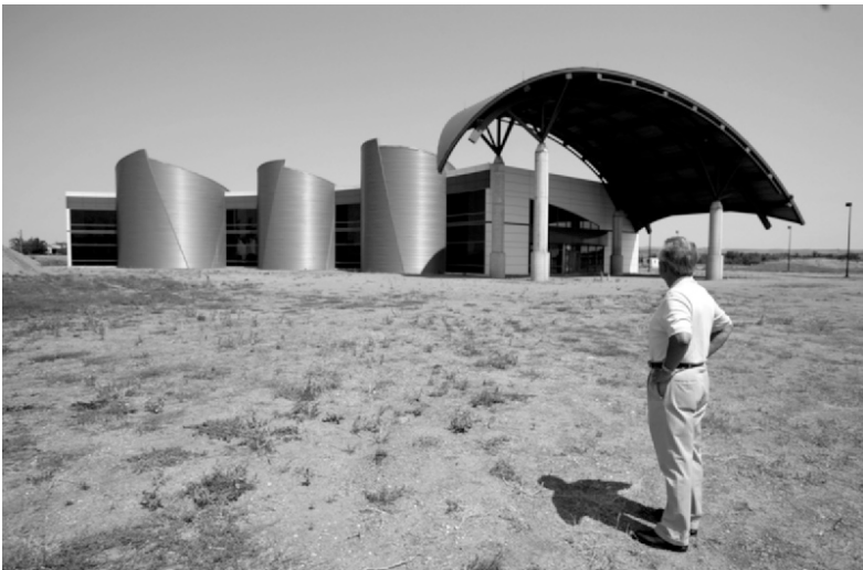
Figure 17 An incomplete Wakpa Sica Reconciliation Place. Richard Rangel, the construction manager at the Wakpa Sica Reconciliation Place, says he is looking for ways to stretch money. © Keith Bedford / The New York Times / Headpress
