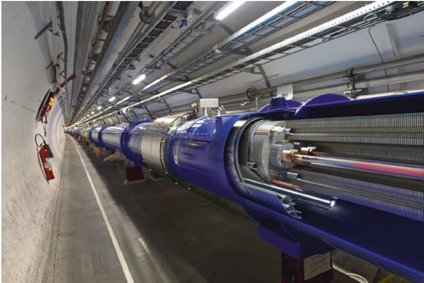
Fig. 1.6 3D cut dipole tunnel montage photo (CERN)
