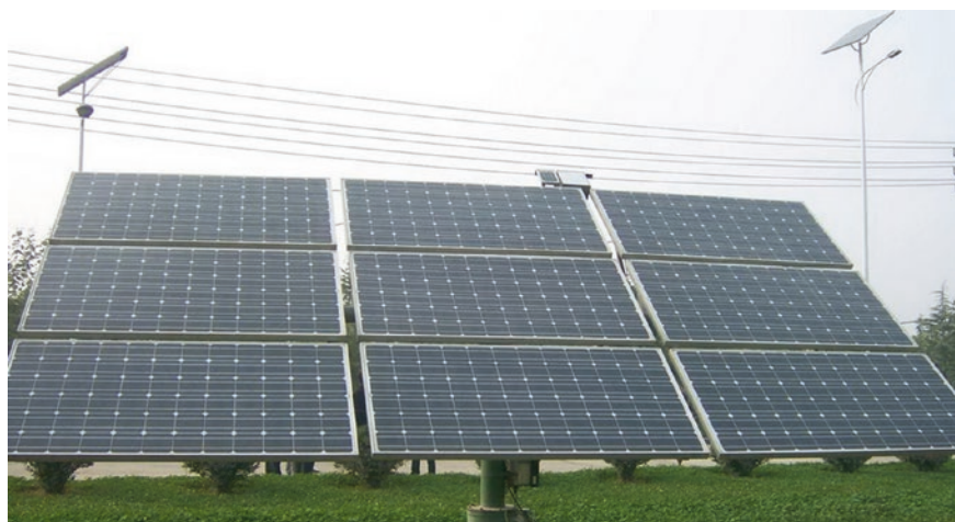
Fig. 5.2 View of a grid interactive solar power plant
