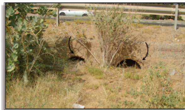
Fig. 10.7 Narrow tunnel filled with sediments in Al-Qaraynah area
