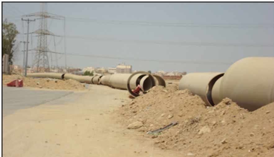
Fig. 10.17 Closed cement pipes to convey water from Wadi Kawes Dam to the old storm-water channel
