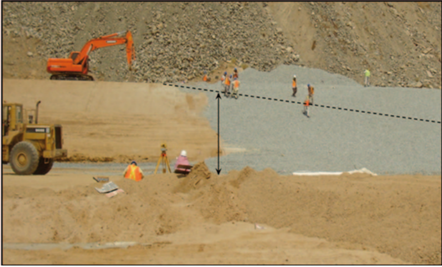
Fig. 10.16 The depth of Omm El-Kheir Dam as appears from Wadi Mriekh side
