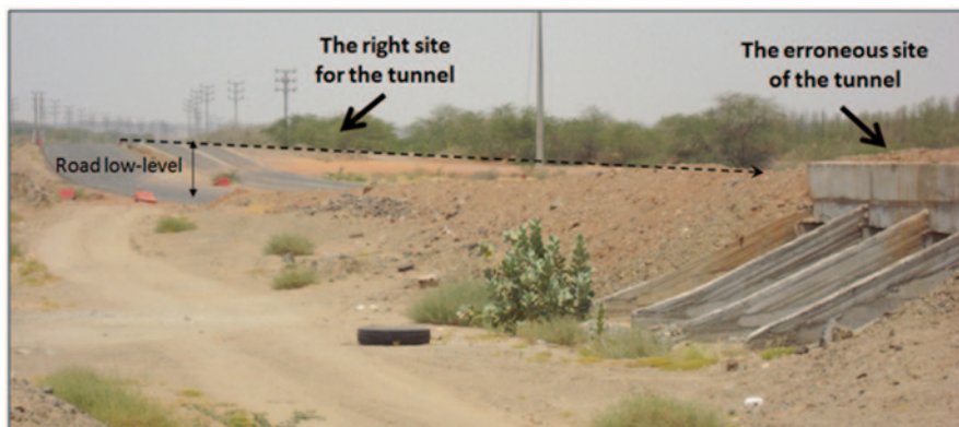
Fig. 10.8 Erroneous tunnel site, which must be at the low-level with respect to the road, but it was located at higher level of the road. Site is located in Al-Fadayalh area
