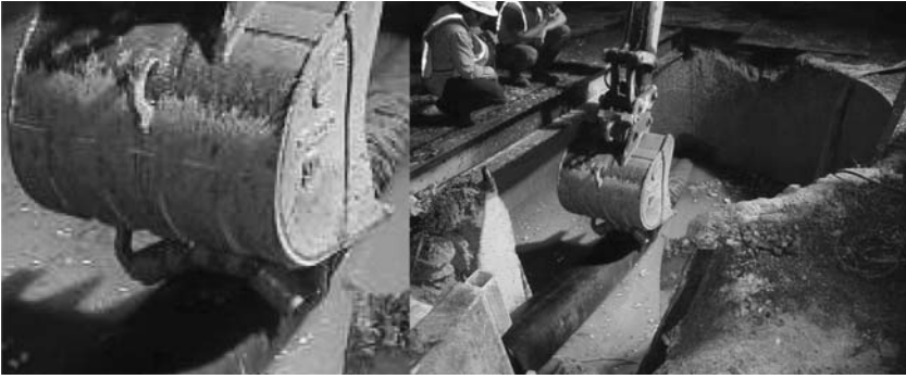
FIGURE 6.20 Protecting the HDPE pipe from grooves using wheels on the bucket. (Source: Handbook of Polyethylene Pipe , 2008.)
