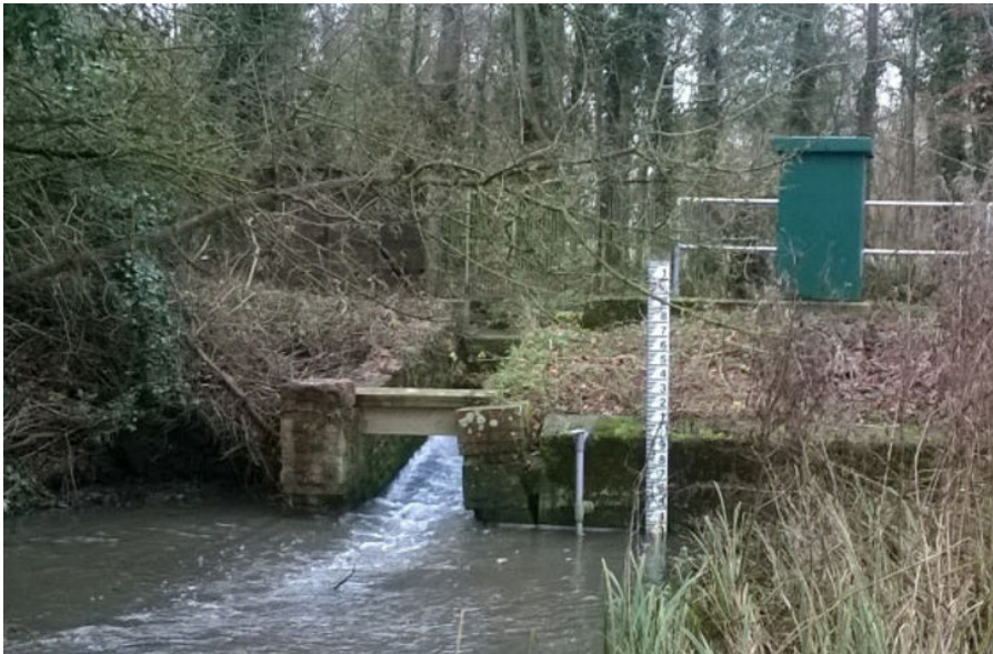
Figure 4.1 An example of water level monitoring.
