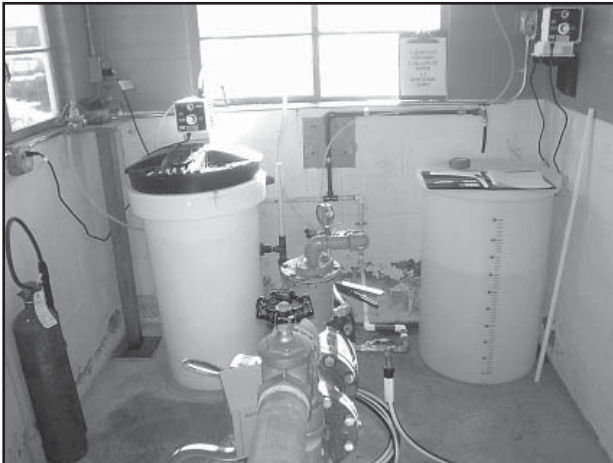
Figure 3-2 Sodium hypochlorite tank (on right) and fluoride saturator in Battle Ground, Washington
