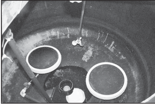
Figure 10-2 Aerators and mixing in hydrous manganese oxide solution tank are used to keep the precipitated manganese in solution prior to injection into the raw water for radium removal.
