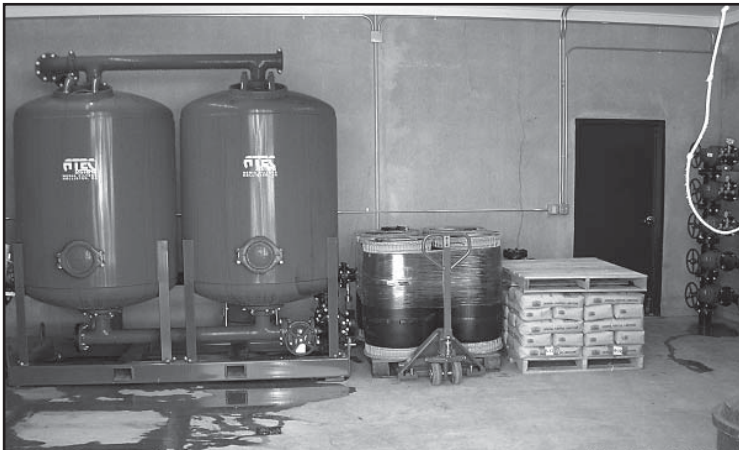
Figure 4-1 A calcite contactor can be a cost-effective way to raise pH for groundwater with low pH and low to moderate alkalinity. These calcite contactors are designed for upflow, so backwashing is not necessary.
