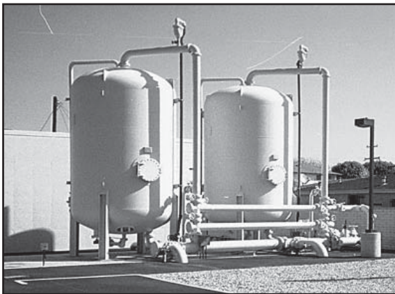
Figure 12-2 These vertical vessels hold GAC, which is used to remove PCE from the groundwater.
