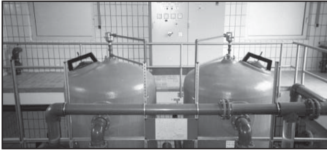
Figure 2-4 Biological iron and manganese removal vessels in Germany
