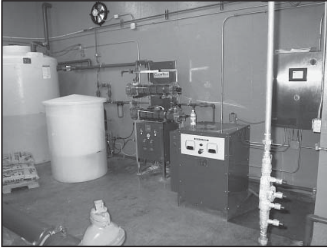
Figure 3-4 On-site sodium hypochlorite generator in Lakewood, Washington
