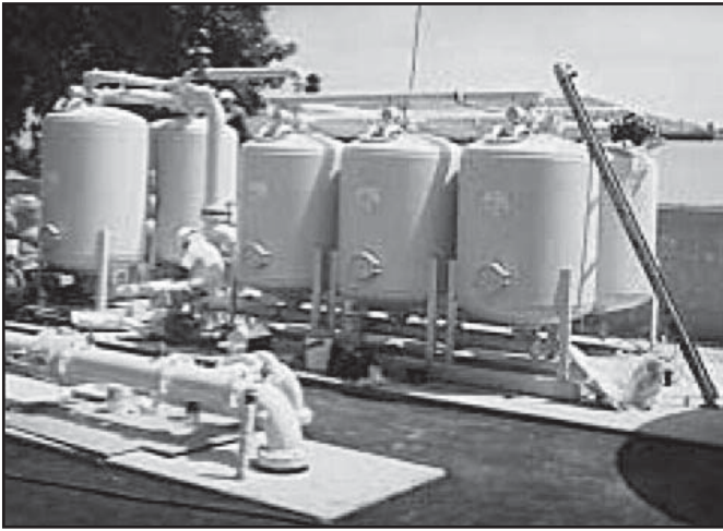
Figure 6-1 The 2003 Juan Plant in Southern California was one of the first US plants to use ferric hydroxide for arsenic adsorption.
