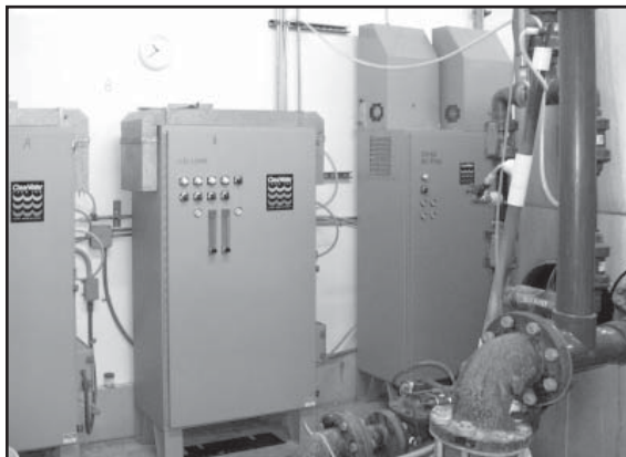
Figure 2-9 Wall-mounted ozone generation equipment in a well building at Camano Island, Washington
