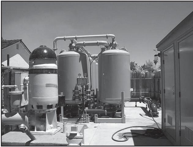
Figure 6-3 This groundwater treatment plant uses preoxidation and ferric chloride addition to remove arsenic in manganese dioxide filters.
