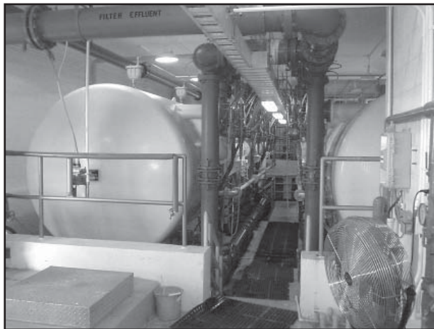
Figure 2-12 Greensand filtration plant in Geneva, Illinois
