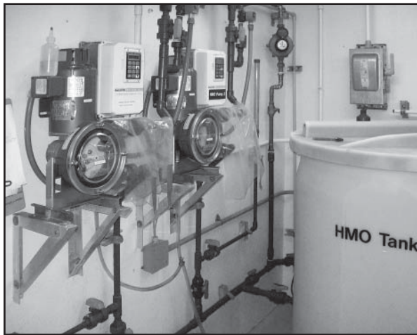
Figure 2-6 Hydrous manganese oxide solution tanks and solution feed pumps
