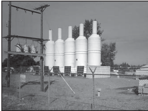
Figure 12-1 These packed-tower air strippers in Tacoma, Washington, are used to strip PCE from groundwater.
