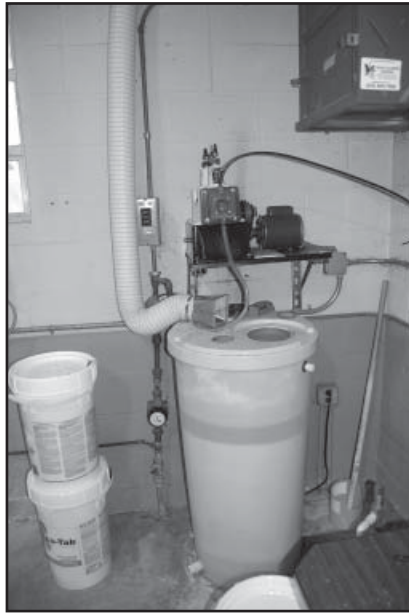
Figure 3-5 A simple venting system keeps chlorine fumes from corroding well house equipment
