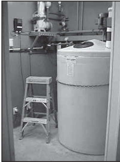
Figure 5-5 Permanganate mixing tank
