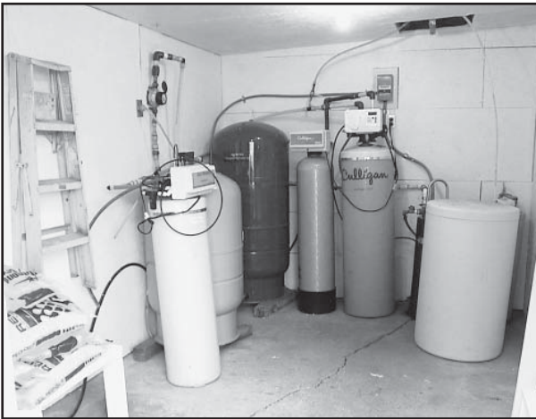
Figure 2-17 Small ion-exchange system installed for iron removal in Washington State
