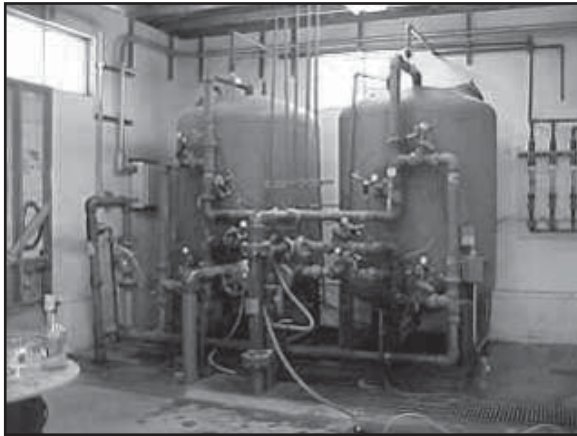
Figure 5-1 Greensand filter system in California
