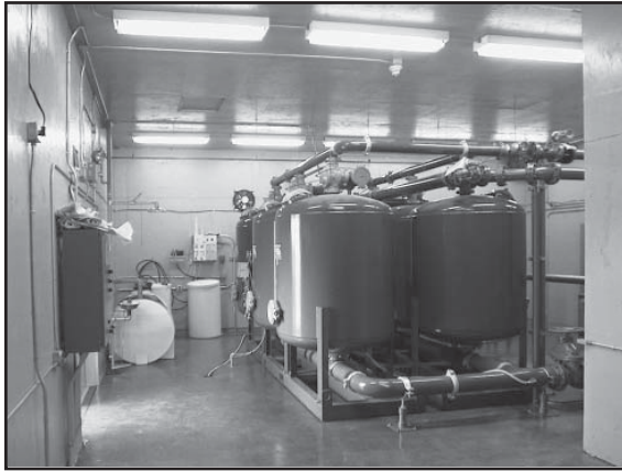
Figure 2-14 Iron and manganese filters at Lakewood, Washington, with filter loading rate of 10 gpm/ft 2 using manganese dioxide media
