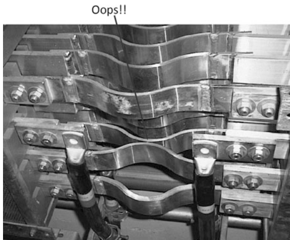
Fig. 4.8 Always expect the unexpected! a wrongly installed cross-bar
