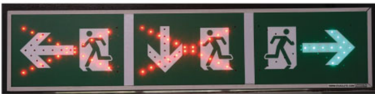
Figure 22.8. The Active Dynamic Signage System used in Trial Series 3 conveying both positive (viable route) and negative (non-viable route) information. For a color version of the figure, see www.iste.co.uk/jacob/safety.zip
